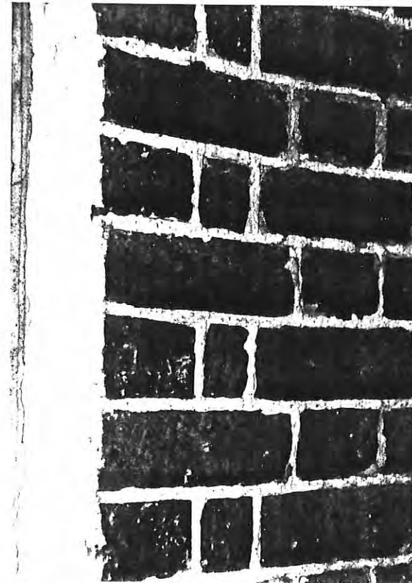
Illustration 22. This damage to the brick and mortar surfaces was produced by sandblasting. The damage is irreversible and will result in the accelerated deterioration of the masonry.
