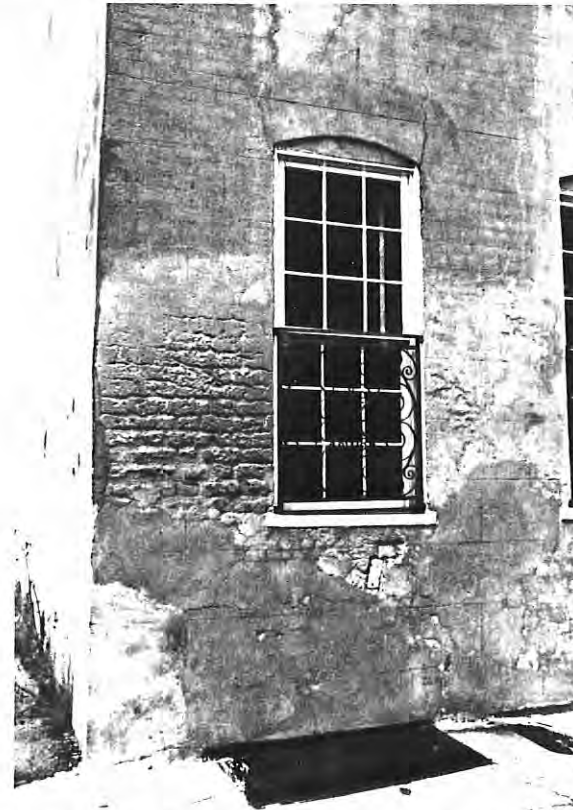
Illustration 11. This illustration of stucco deterioration shows the affects of using dense cement stucco in the repair of porous masonry. The lower wall has been previously repaired with portland cement. The moisture within the masonry has been driven higher in the construction, beyond the original area of deterioration.
