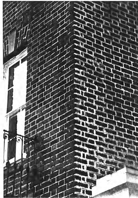
Illustration 13. Seemingly small changes in the size or tooling of the mortar joints can produce dramatic changes in the appearance of a structure. Here, the use of a modern joint tool for the repointing of the side elevation produced an unfortunate alteration to an otherwise exceptional exterior.
