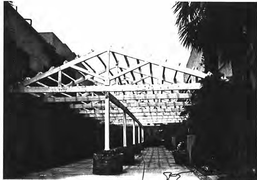
Illustration 25. The exposure of wood elements to weathering, as shown here, requires the installation of additional flashing details and the maintenance of the protective coatings. This example of roof trusses has now been removed due to accelerated deterioration.
