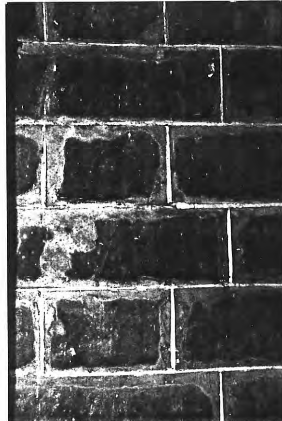
Illustration 5. This variation of the ribbon joint is similar to tuck pointing. A brick colored mortar has been rubbed into the spaces between the brick edges and the ribbon joints.
