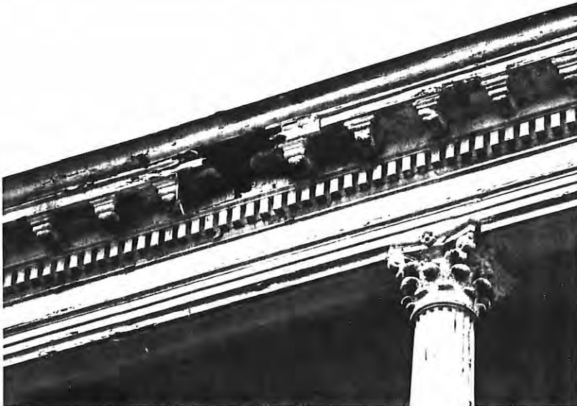
Illustration 23 and 24. The durability of wood construction and its protective coatings is dependent upon the maintenance of the roof, flashing and gutter systems. These leaking built in gutters are responsible for the deterioration of the wood and the failure of the paint.
