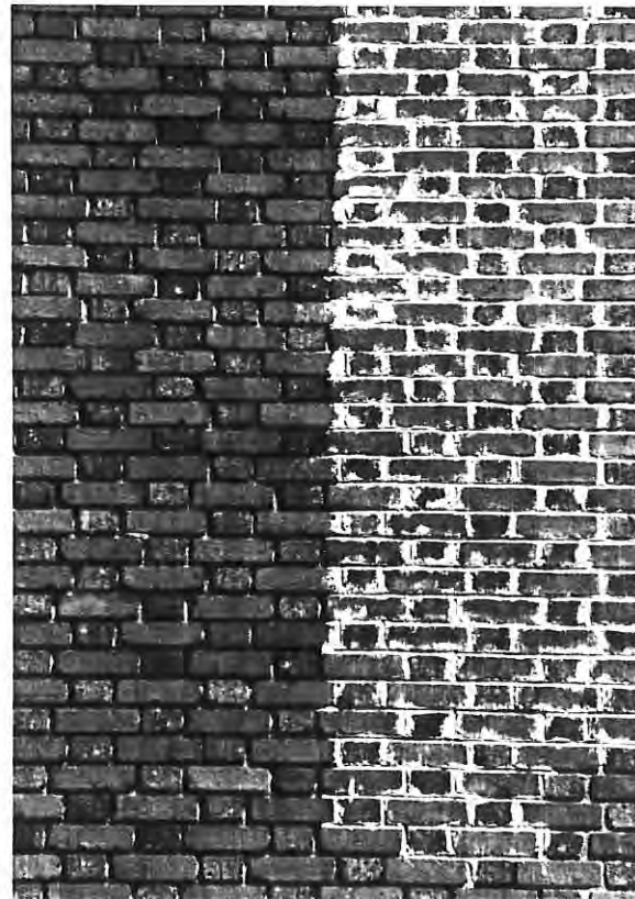
Illustration 17. This early twentieth century example of recessed mortar joints has deep shadow lines. The repointing to the right altered the original detailing by filling the joints. The alteration provides no additional weather resistance to the construction. The actual effect of the repair will likely be an increased need for maintenance of the repair area due to the shallow depth of the new pointing.
