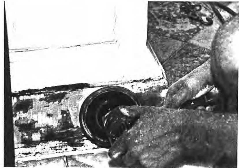
Illustration 26. The use of disc sanders and other abrasive tools to remove paint account for the greatest loss of architectural details among Charleston's wooden structures.
