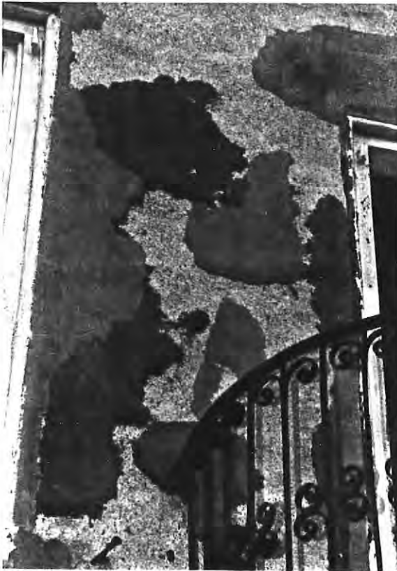
Illustration 12. This illustration of stucco repairs shows the original lime stucco, a dark natural cement stucco from the period of the 1886 earthquake repairs and grey portland cement stucco repairs of the twentieth century. The relatively porous lime and natural cement stuccoes are performing well. The denser portland cement is accelerating the deterioration of the surrounding stuccoes.
