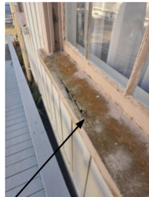
Weathered window sill.
