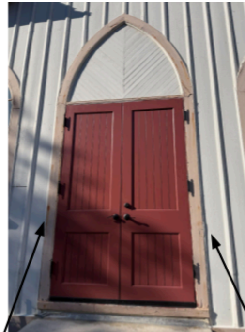
Patina from corrosion on door frame.
