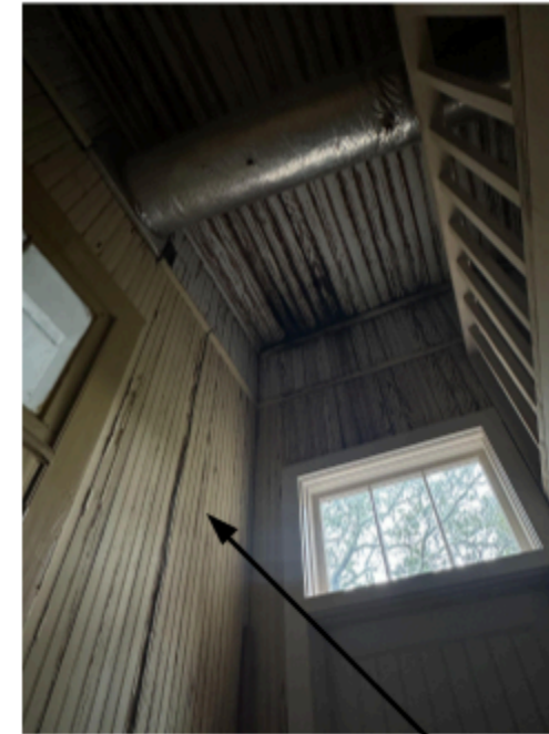
Chipping and breaking throughout.
