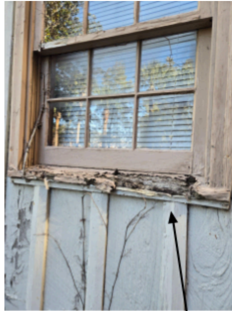
Rotten window sill.
