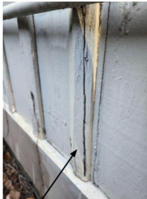
Cracking on siding.
