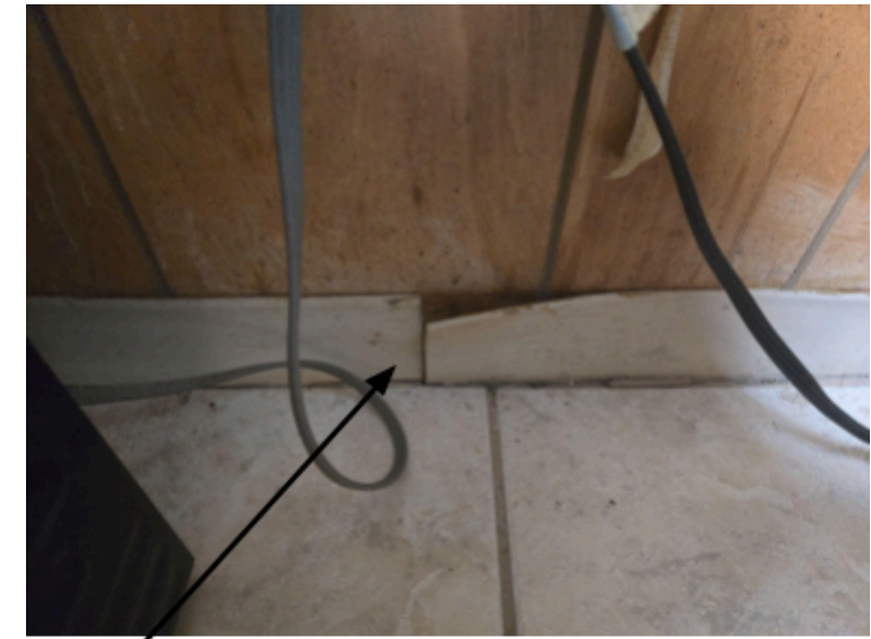
Baseboard detaching from panelled wall.
