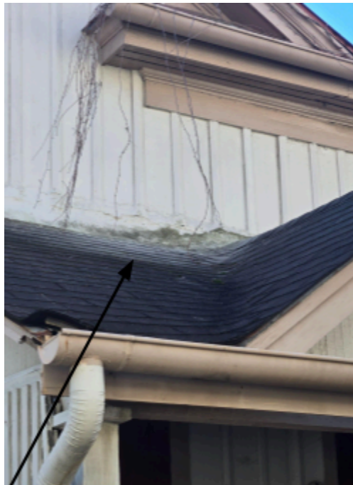
Mold at porch to siding connection.
