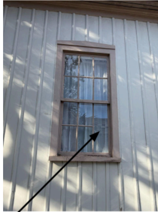
Missing window muntin.
