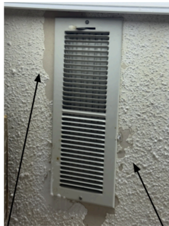
Surface treatment failing around vent.
