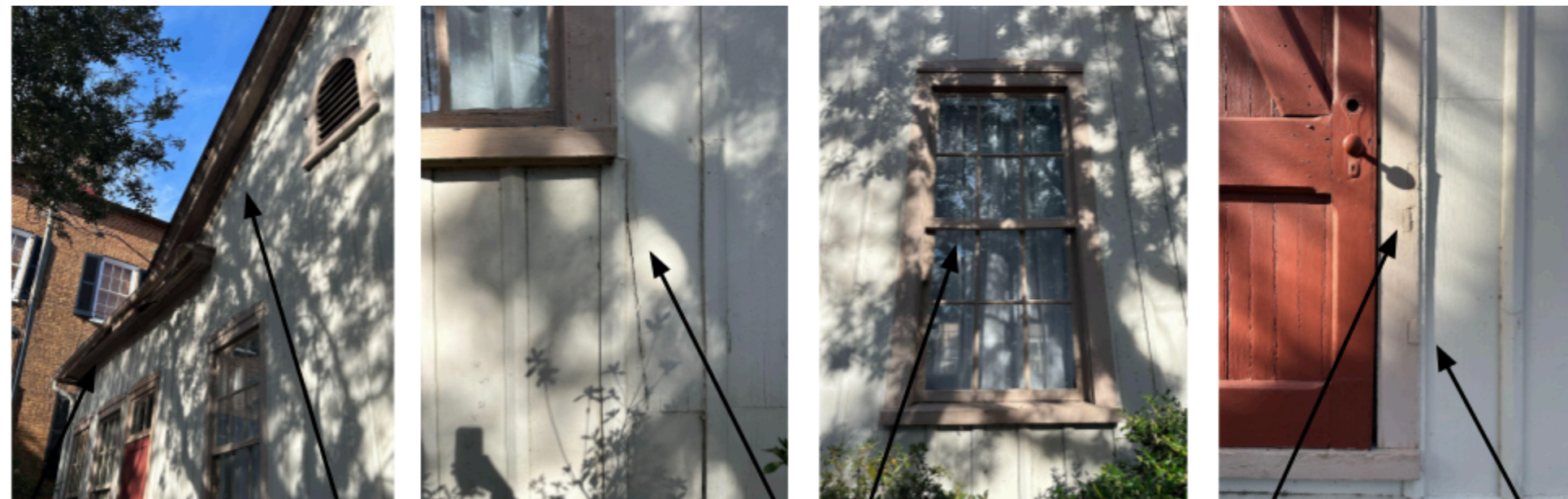
Vegetation on the eaves.
