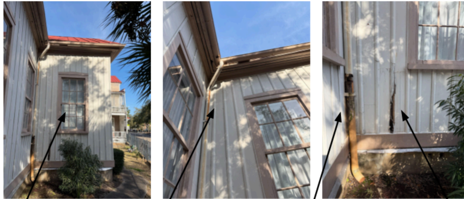
Sagging window sash.
