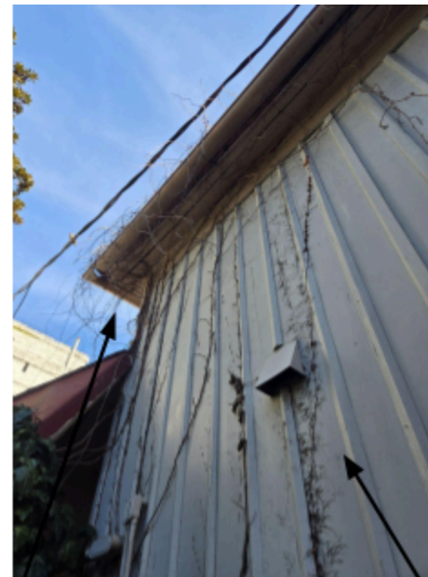
Vegetation on siding and in eaves.
