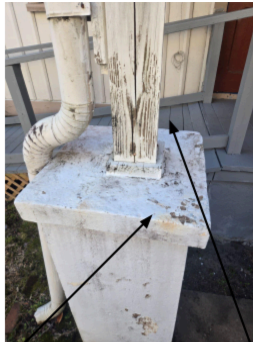
Water damaged support post and base.
