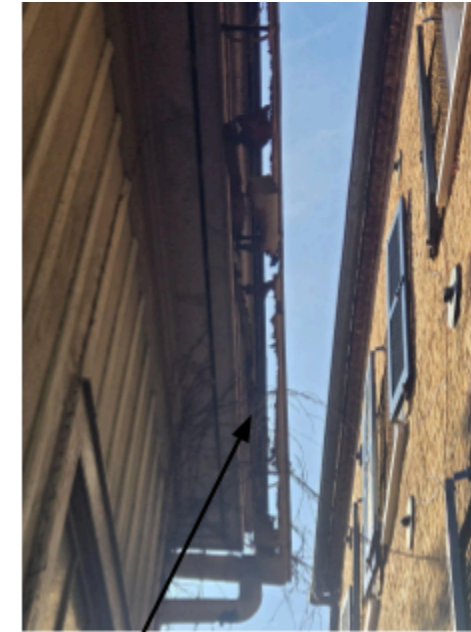
Rusted out gutters.
