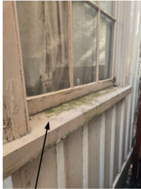
Mold on window sill.
