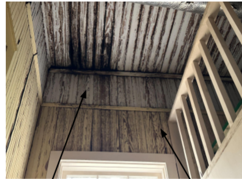
Surface Deterioration throughout, water damage.
