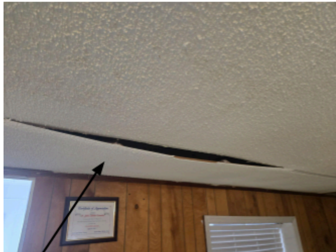
Drywall sheet detaching from ceiling joists.
