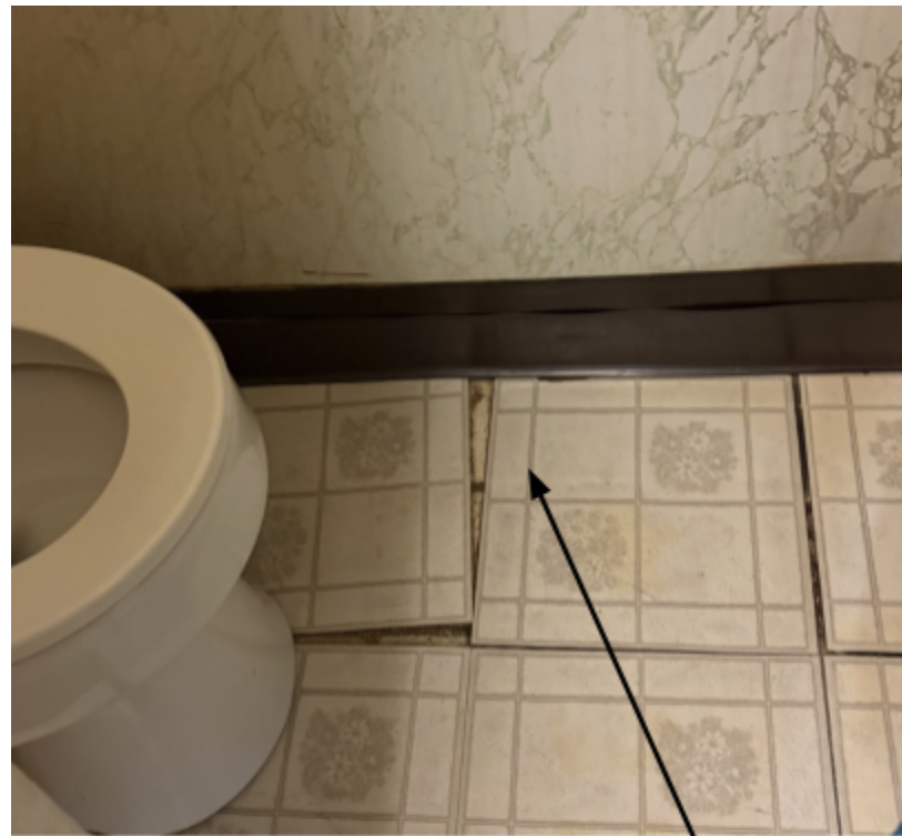
Delamination of laminate flooring.
