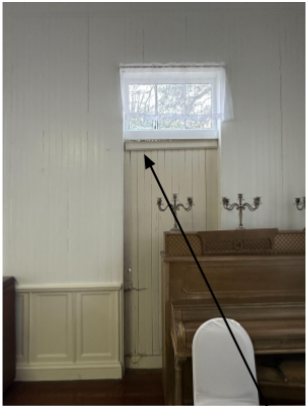
Structural drop above door frame.
