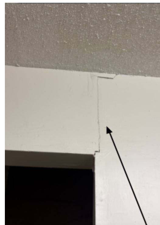
Structural crack over door opening on east elevation.
