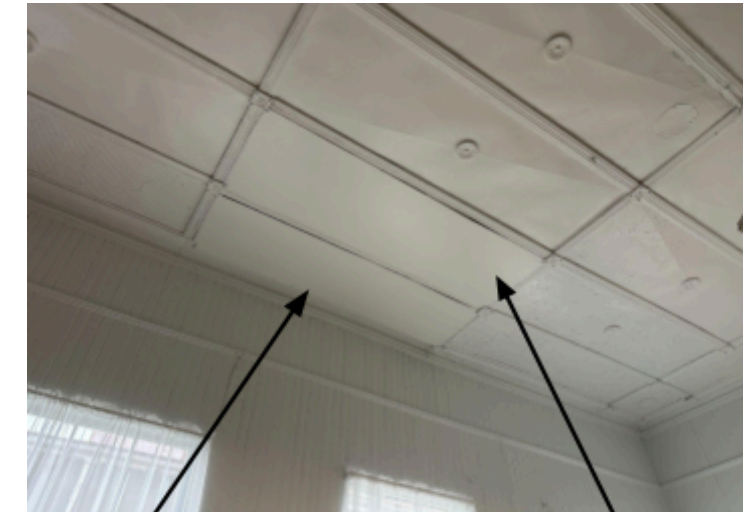
Two patched wood panels in tin ceiling.
