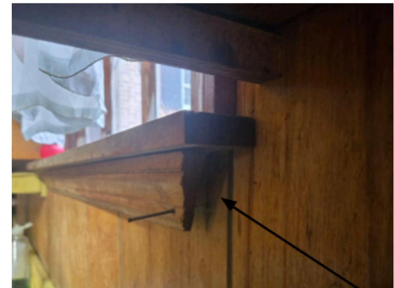
Trim under window sill detached from wall.
