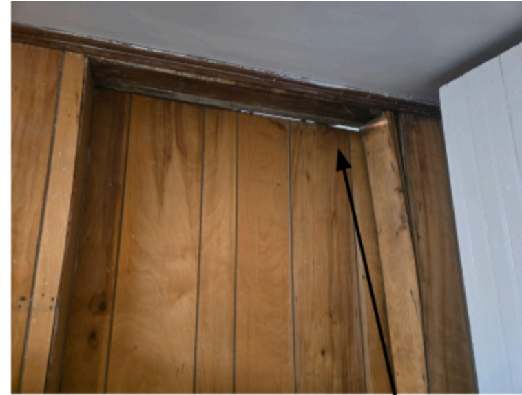
Gap over door opening.
