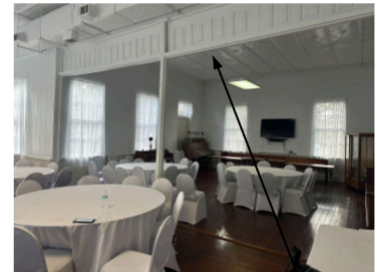
Structural sagging in partition wall.
