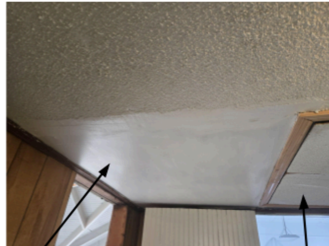
Ceiling patch, and wear on attic door from assembly hall door scratching.
