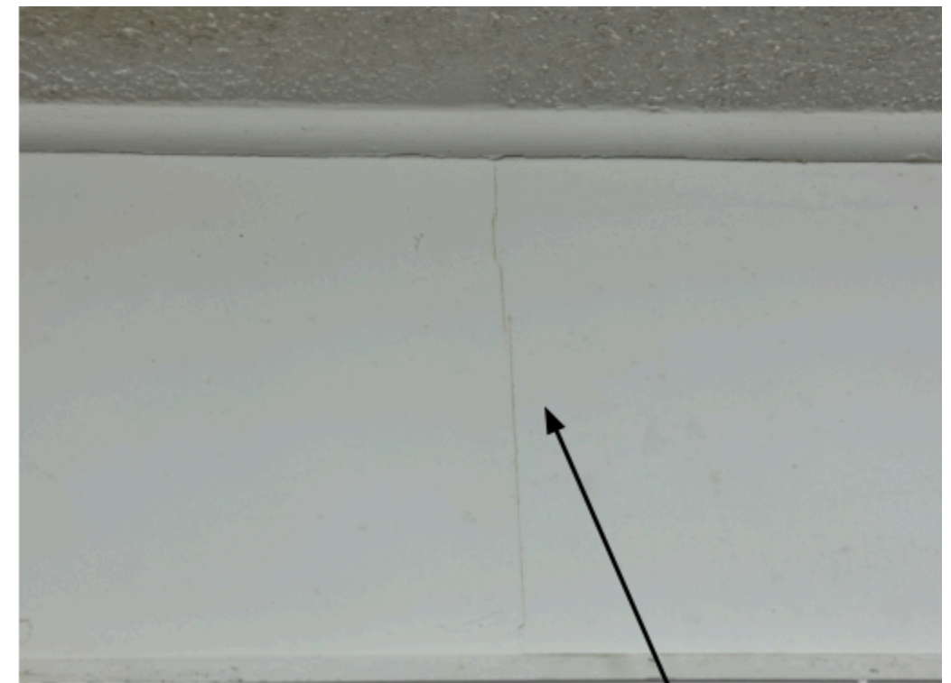
Structural crack near ceiling.
