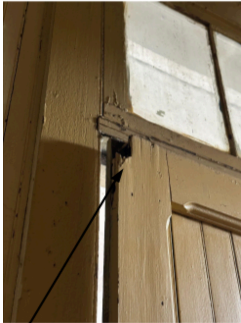
Water damage on door corner.
