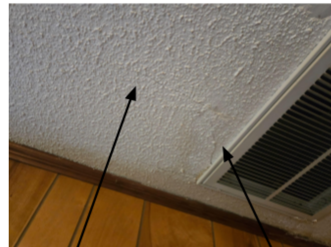
Crack in surface treatment.
