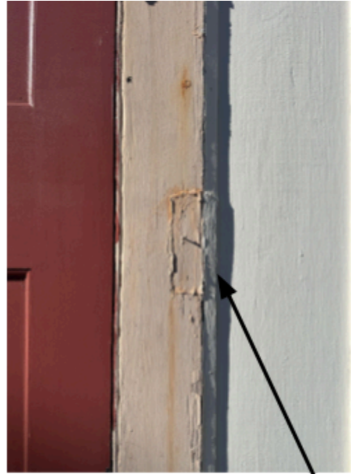
Patching on door frame.
