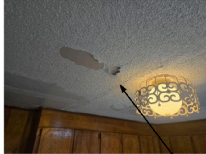
Popcorn surface treatment failing.
