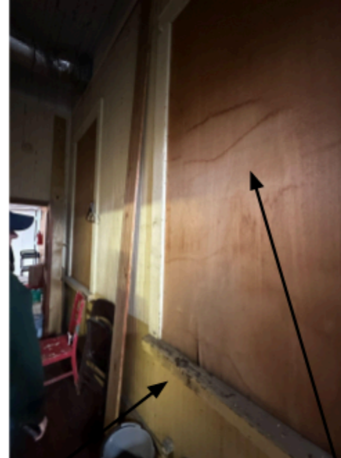
Water damaged sill and infill board.
