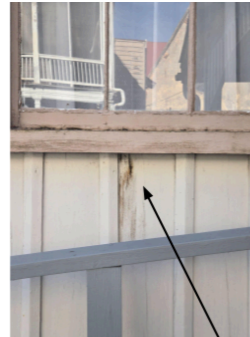
Rot under window opening.
