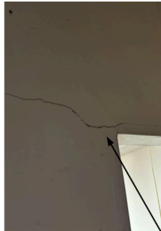
Structural crack near door opening.
