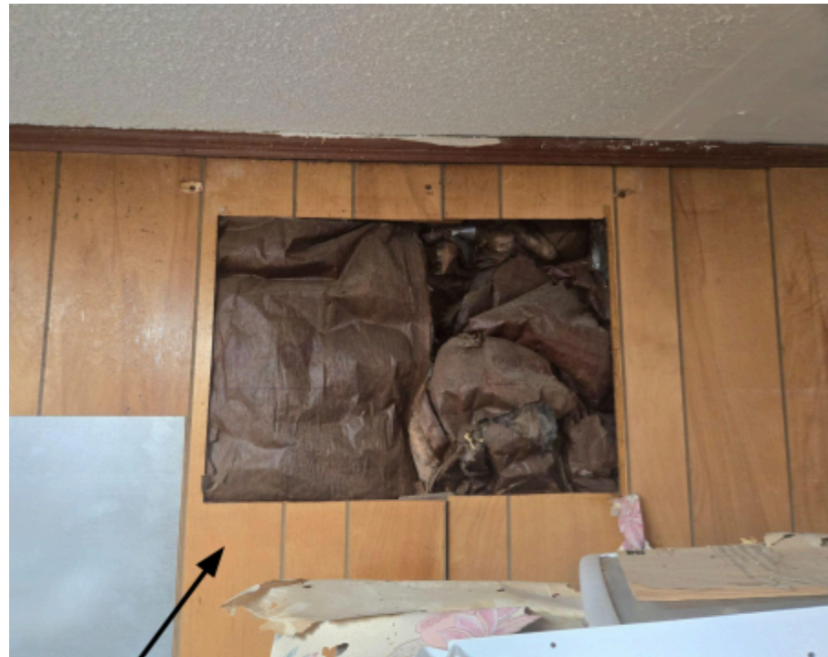
Hole in paneling, insulation visible.
