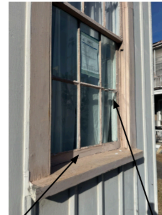
Water damage to window frame.
