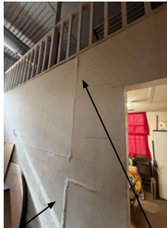
Surface deterioration throughout.
