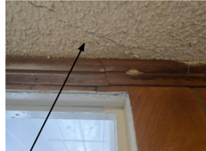
Crack at ceiling and wall connection.
