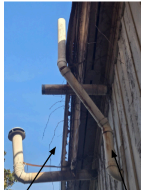
Rust and Patina on Gutters.
