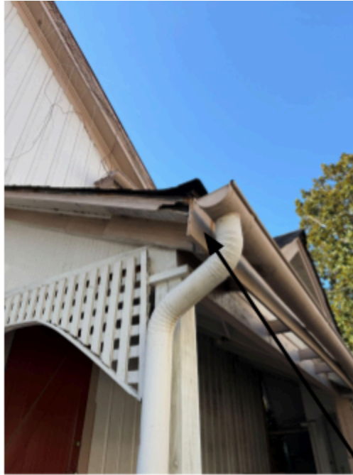
Water intrusion on porch overhang.
