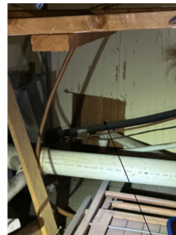
Hole in wall above bathrooms.
