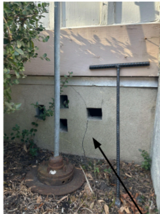
Structural foundation cracking.
