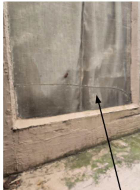
Cracked glass in window.
