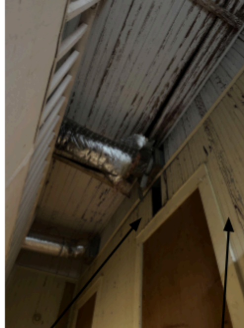
Surface deterioration, Hole in wall under HVAC duct.
