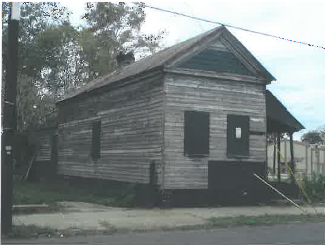
Figure 11: 199 Jackson Street, modern plywood covers windows, doors, and holes in clapboard. Screen door leading from the street to piazza is missing. Photo by the author, November 2009.
