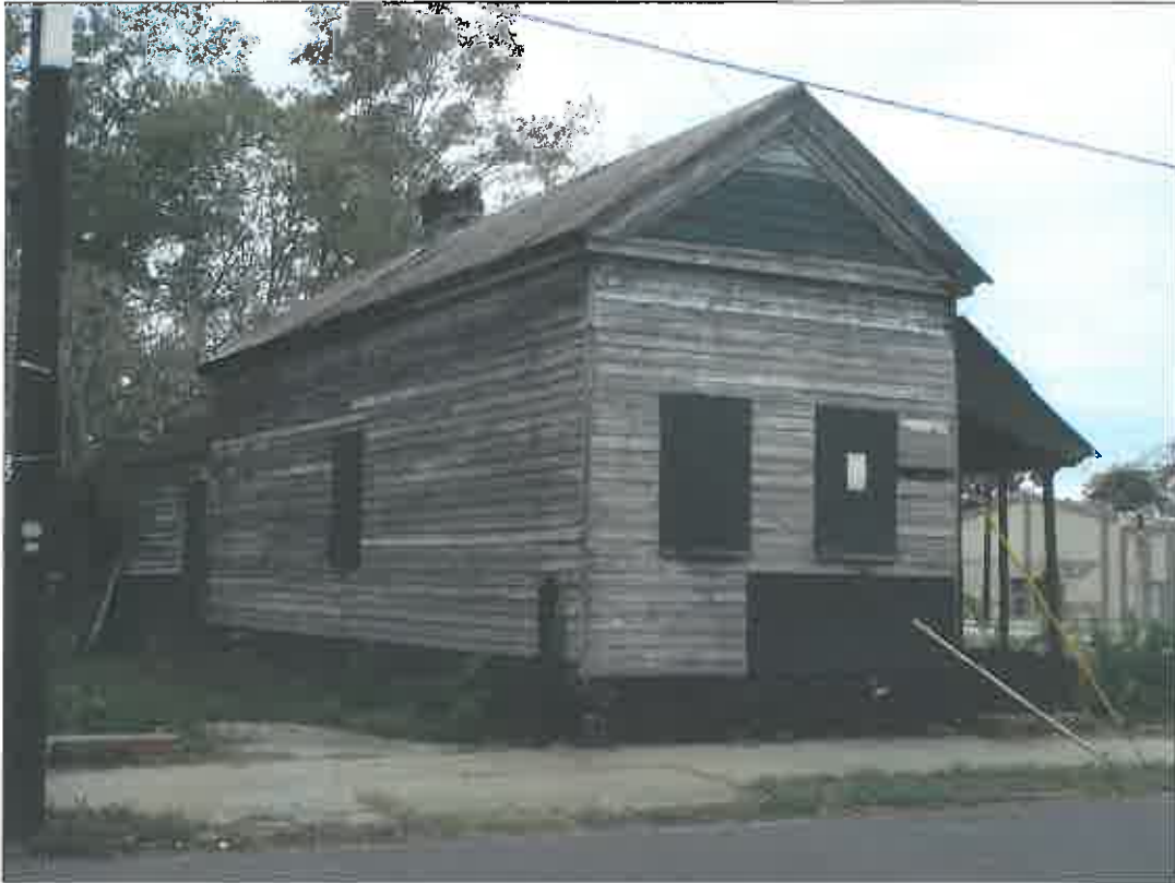
Figure 20: Plywood is used for stabilization and to cover all exterior openings, as well as prevent access under the buildings. Photo by the author, November 2009.
