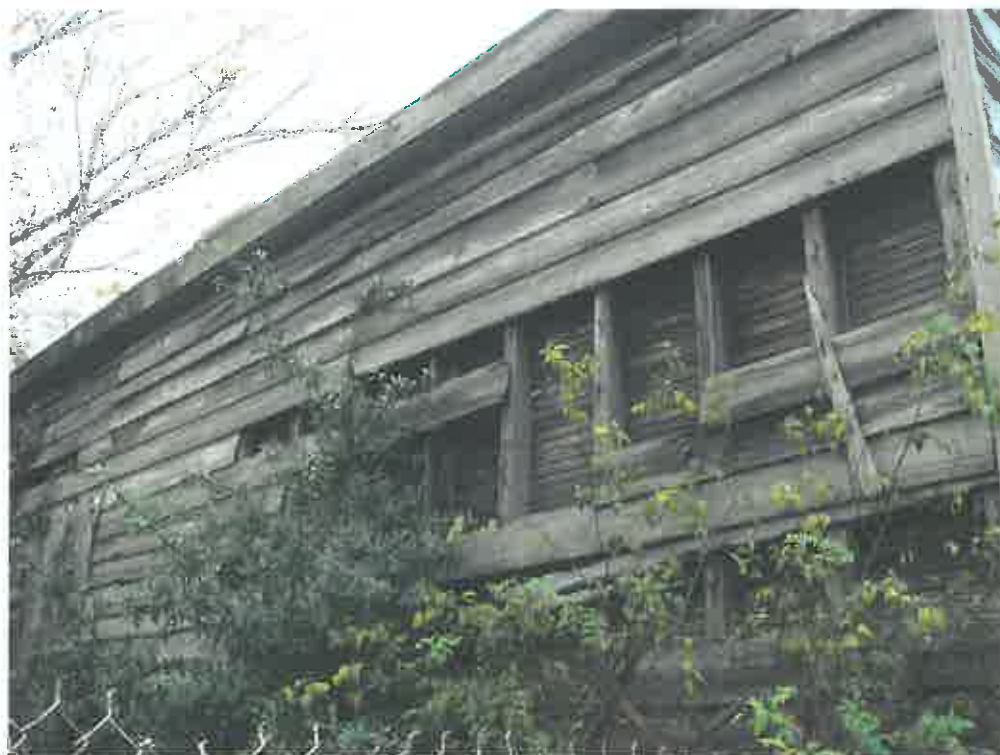
Figure 12: Missing clapboard on east side of 193 Jackson Street. Photo by the author, November 2009.
