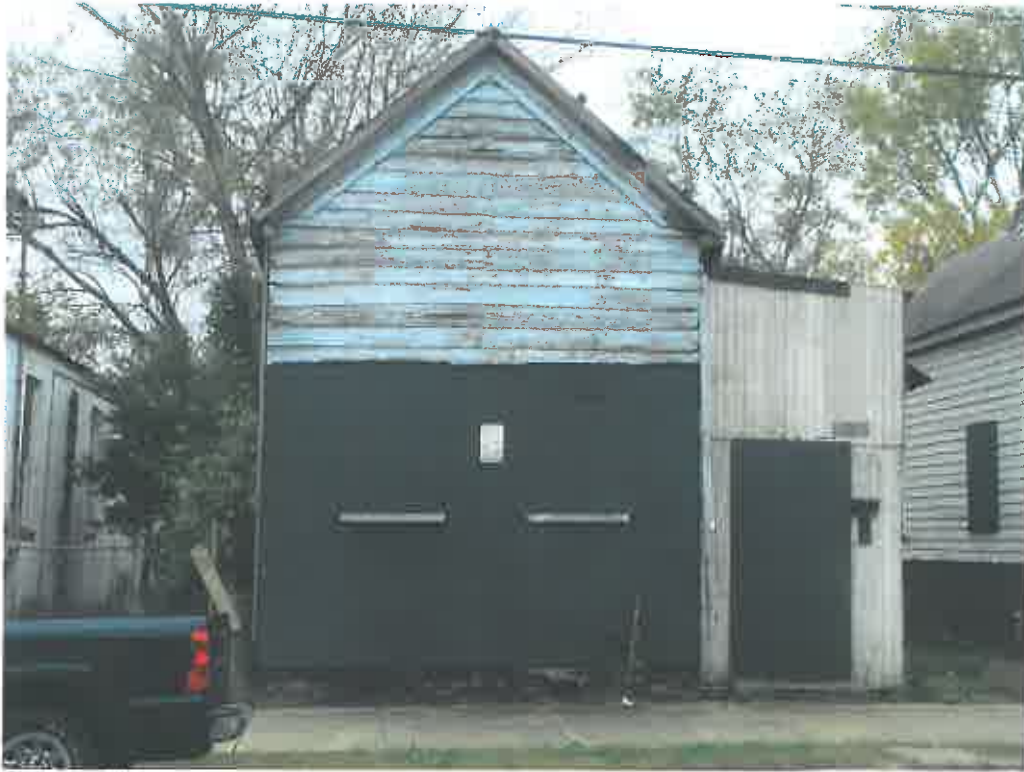
Figure 8: 193 Jackson Street, missing bottom portion of pediment enclosure. Mismatched vertical clapboard surrounding door leading to piazza. Photo by the author, November 2009.
