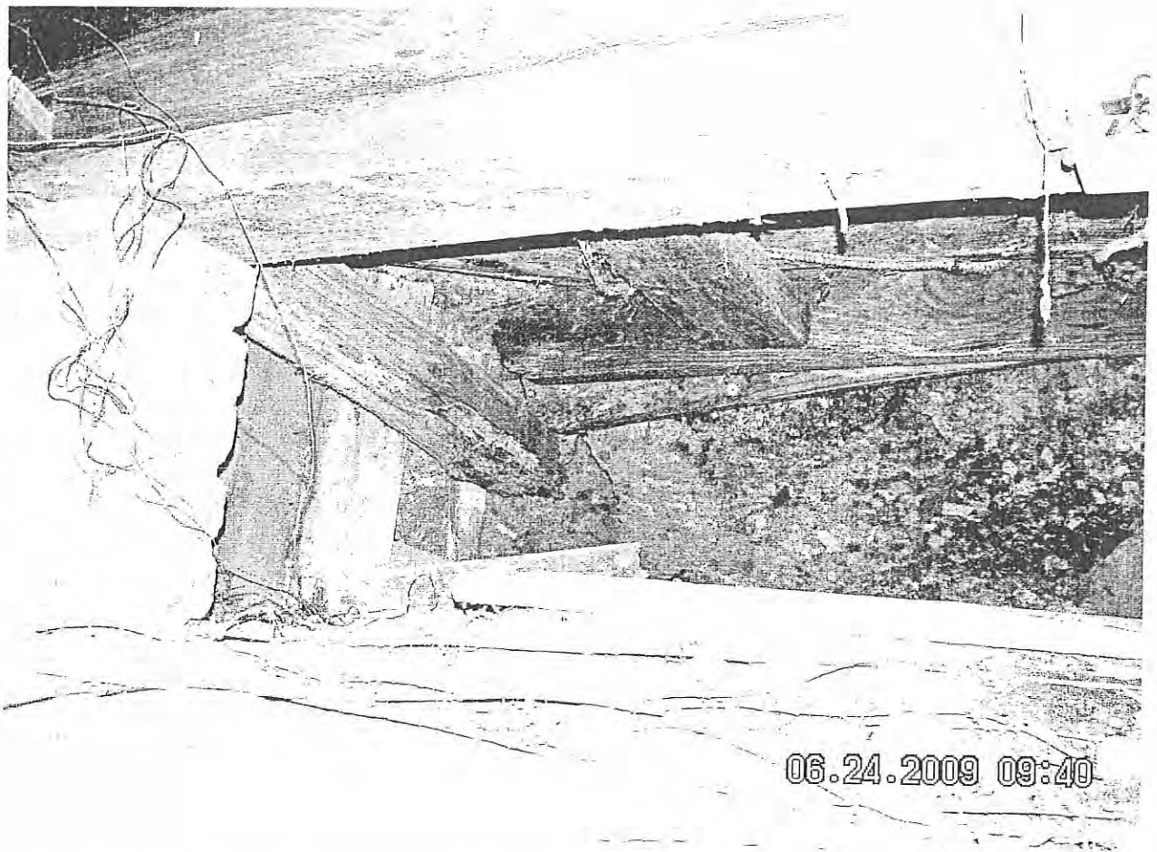
View under front porch - note there are no foundations under bay window area.
