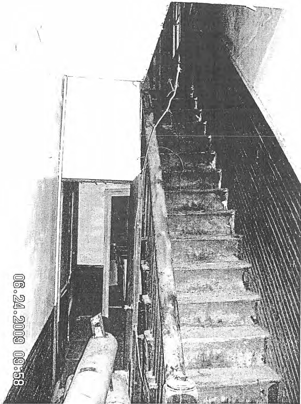
First Floor Hallway - note extremely narrow stair
