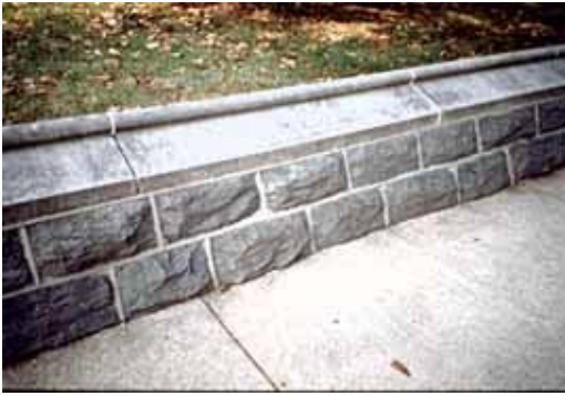
Caulking was inappropriately used here in place of mortar on the top of the wall. As a result, it has not been durable. Photo: NPS files.
