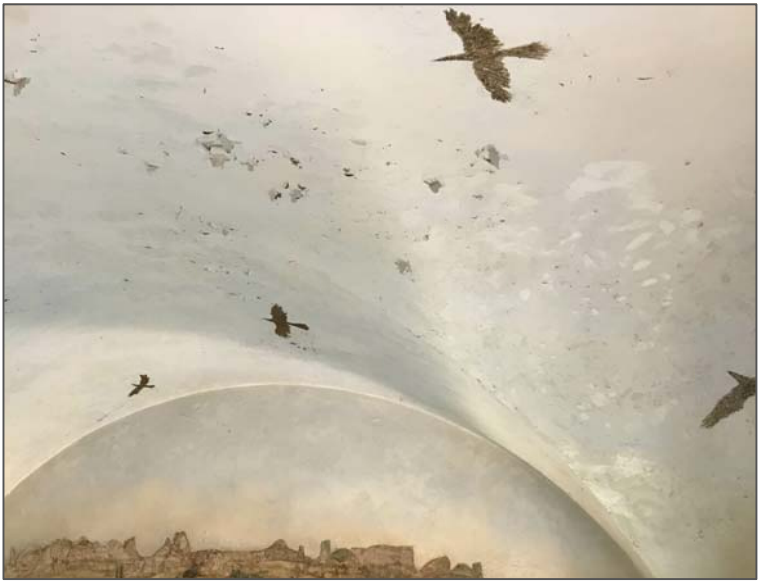
Ceiling: note large areas of peeling paint, different paint sheens and old repairs.
