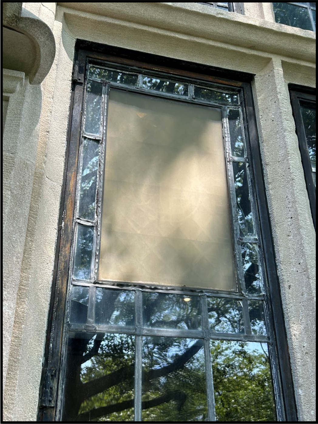
FIGURE 3: Detail of warped/mangled lead around metal box, view from exterior
