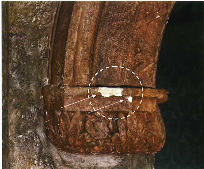
North Elevation—Approximate Grid Location #20 Losses around the northwest archway. Relatively large losses of delicate areas caused by physical contact.
