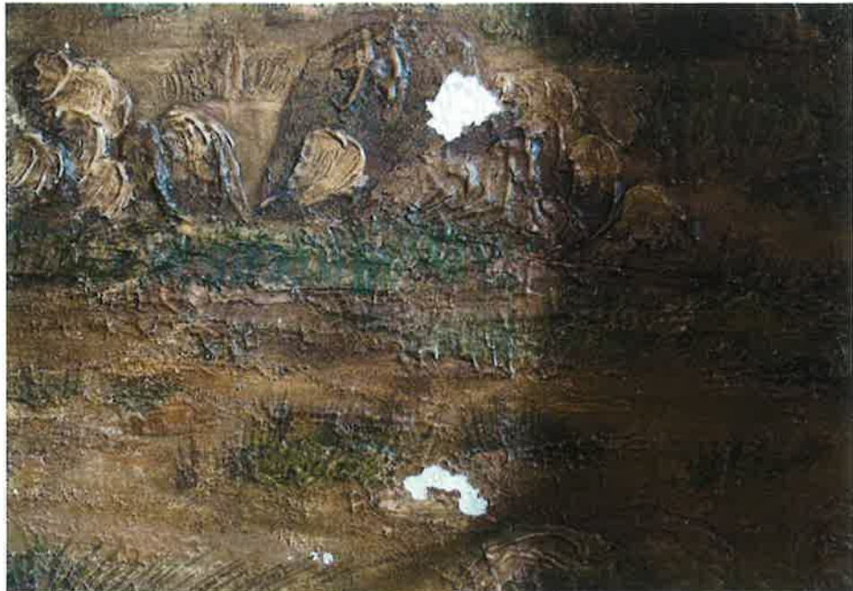
East Elevation Approximate Grid Location #15 Large areas of recent loss that have expanded since 2007
