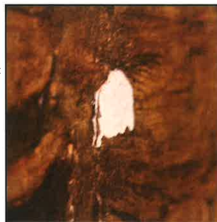
Breakfast Room 2012. Detail of detachment. Gesso layer has detached from plaster.
