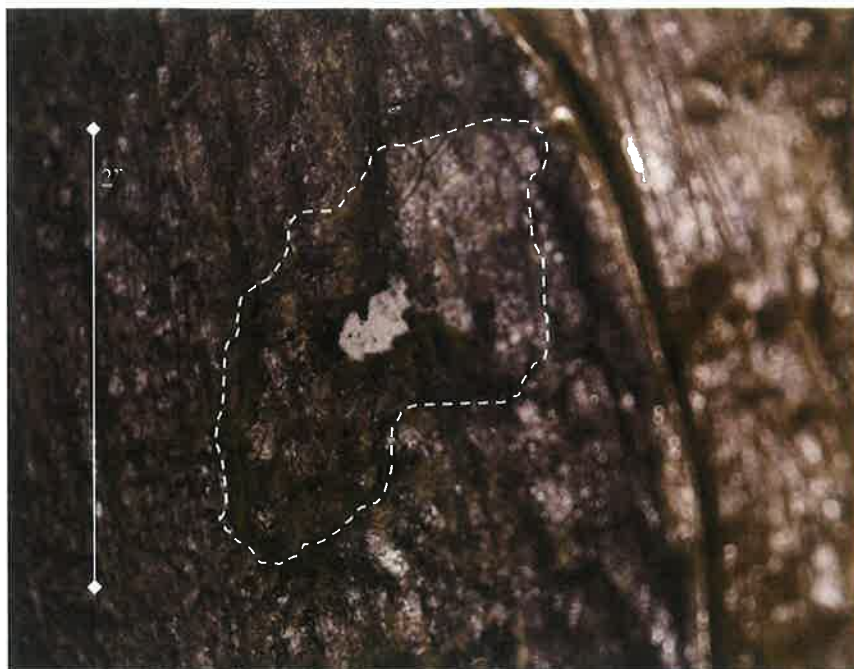
North Elevation—Approximate Grid Location: 16 Typical condition: note highlighted large pocket of highly unstable detached paint and gesso around a section of loss. The outlined area has detached from the plaster.
