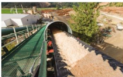
One energy-saving idea was to simply replace the mill's 200-hp pneumatic chip blower with a 15-hp conveyor.
