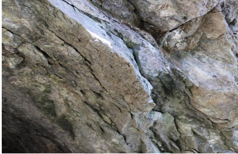
Figure 5: Highly weathered and fractured rock around the Cave portal.
