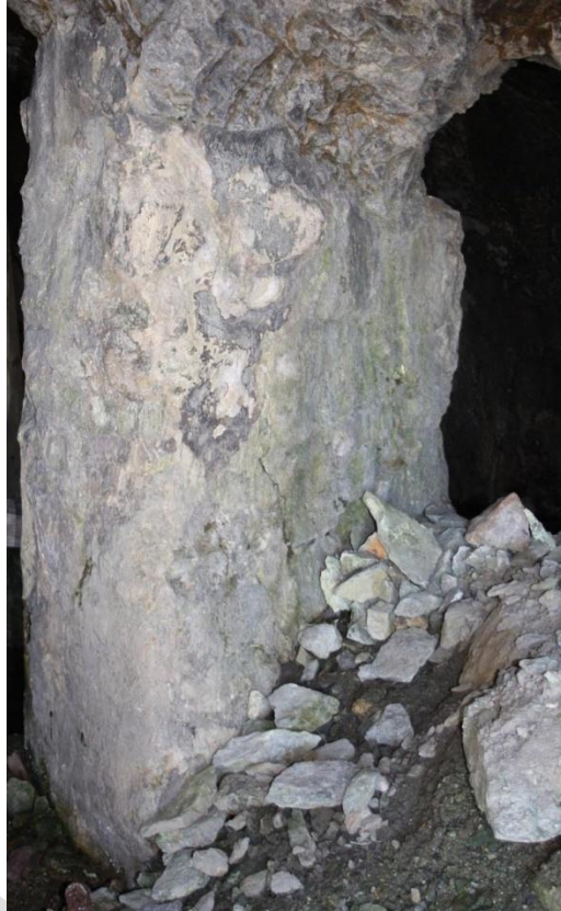
Figure 7: Rock debris/spalling on the floor near rock pillar
