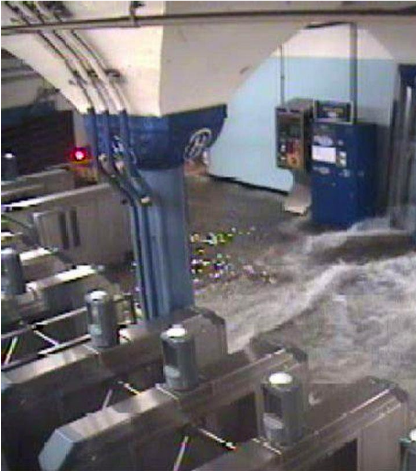
<img class="aligncenter size-full wp-image-38577" title="Floodwaters from Hurricane Sandy rush into the Port Authority Trans-Hudson's (PATH) Hoboken, New Jersey station through an
