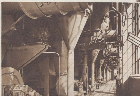
Batteries of new Thermalo roasters, largest batch coffee roasters in the world, supplied by Jabez Burns, are seen in operation above. After roasting, coffee is spouted immediately to the coolers below the operating platform.
