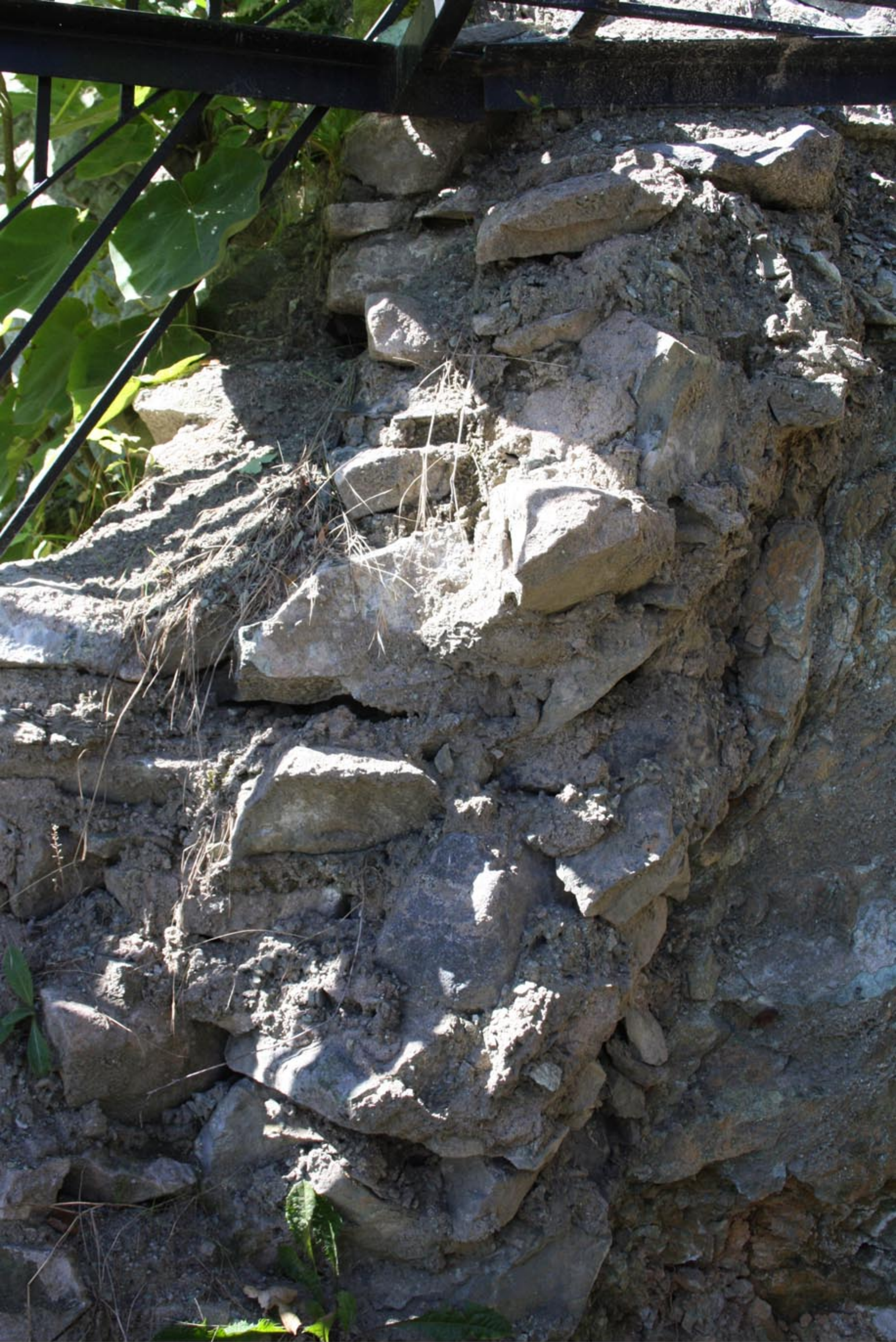
039 Sybil's Cave, Hoboken NJ 9-21-2010 View of SE face at entrance circa 8 feet from ground where ironwork connects
