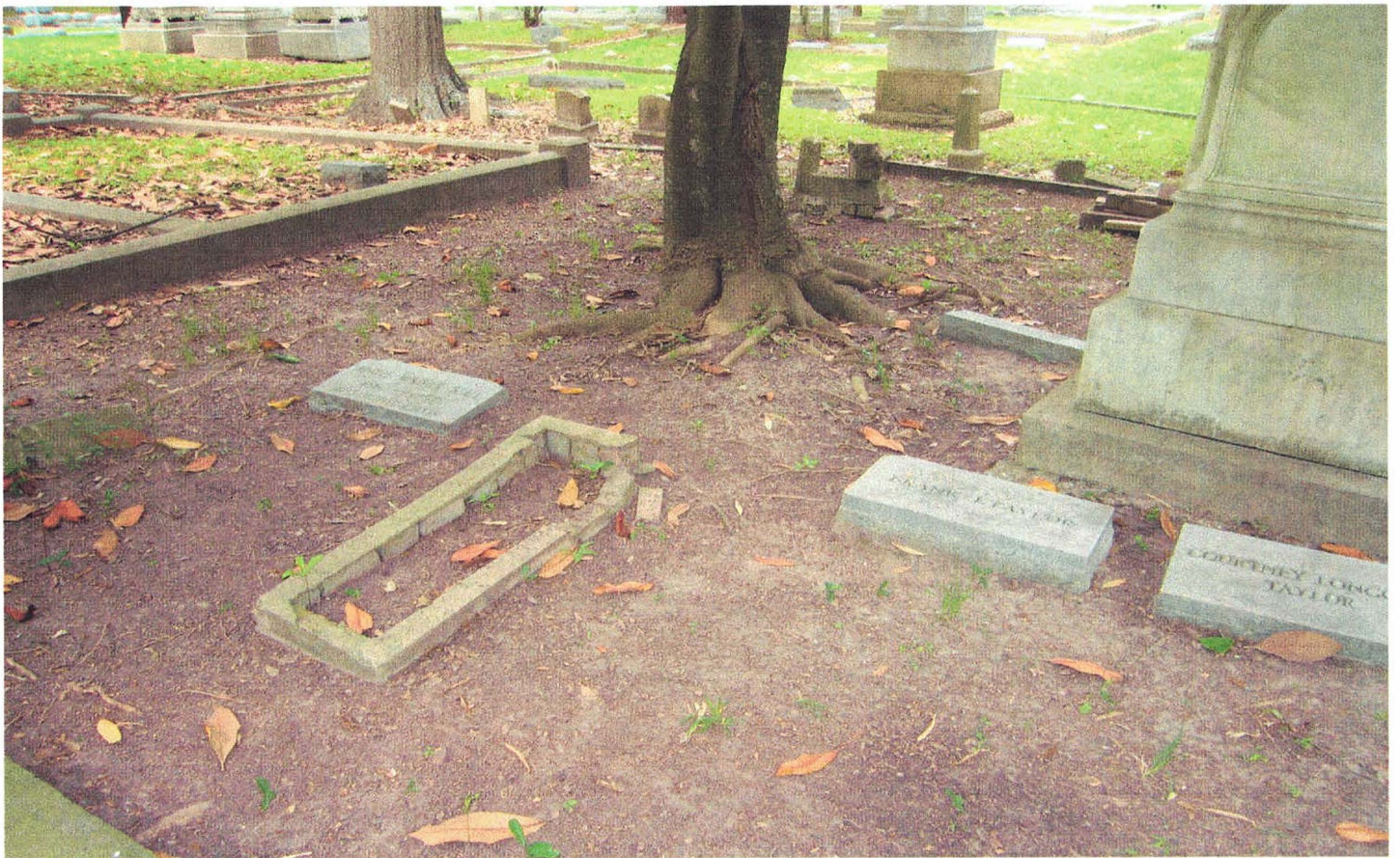
Before restoration, most of the stucco was missing from a small cradle.
