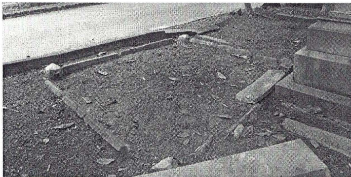
BEFORE: The marble coping in the southeast corner of the lot is badly damaged but recoverable.
