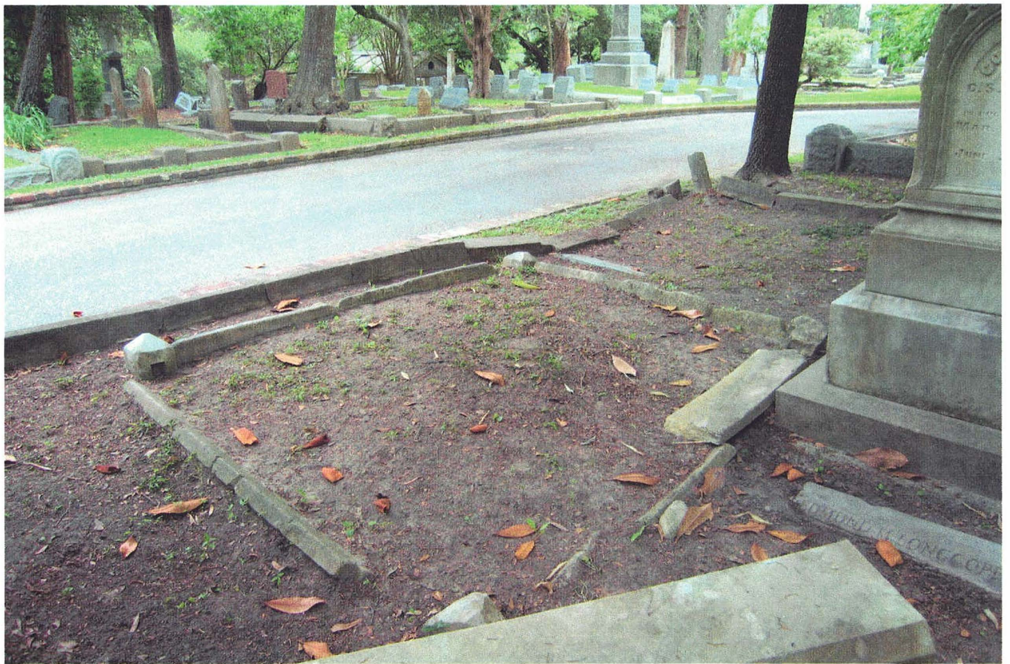
Before restoration, a small marble coping within the lot was badly damaged and partially missing.
