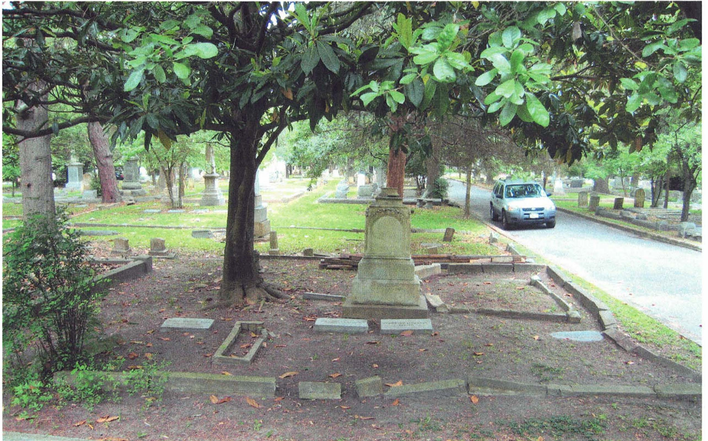
Before restoration, much of the coping (stucco over brick) was missing and what remained was damaged beyond repair
