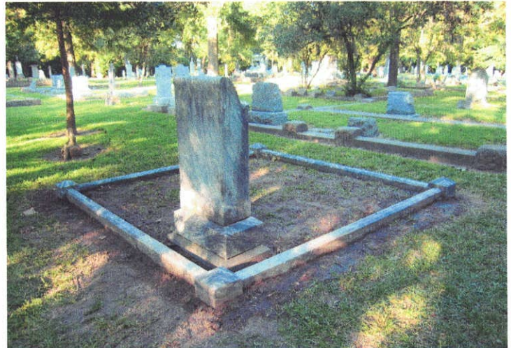
AFTER: The missing piece of the coping has been recovered and the four posts and the entire coping has been leveled and reset on a new foundation.
