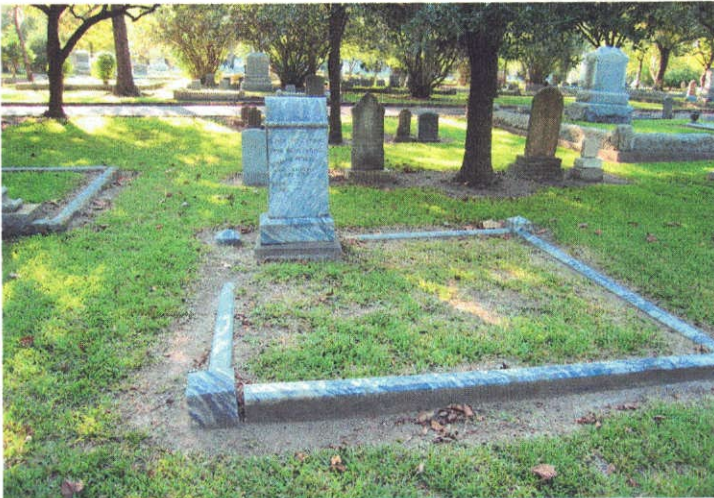
BEFORE: The marble coping has sunk and is buried on the southwest corner. The beam of the coping is cracked behind the monument and a section approximately 2' long is missing.
