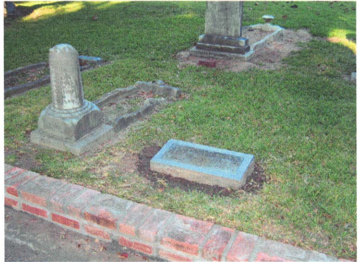
AFTER: The marker has been raised, leveled and reset on a new foundation
