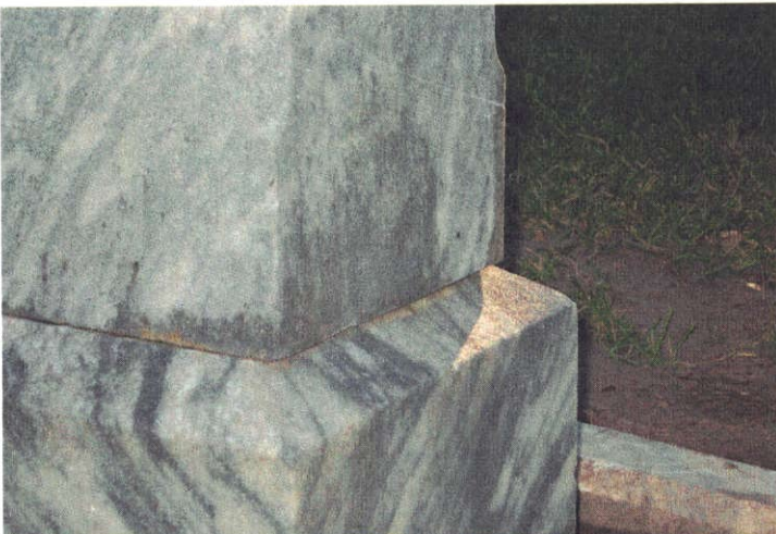
BEFORE: The monument is sliding on its base and overhanging the northwest corner approximately 1".
