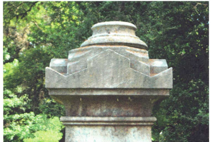
AFTER: The piece on top of the marble monument is loose and has shifted. Investigate whether the marble vase in the granite cradle is actually the finial of the marble monument.
