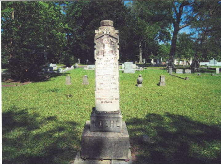
Before: The monument is almost plumb, but is not on a proper foundation. It is sitting on concrete pavers, leveled by small stones used as shims.
