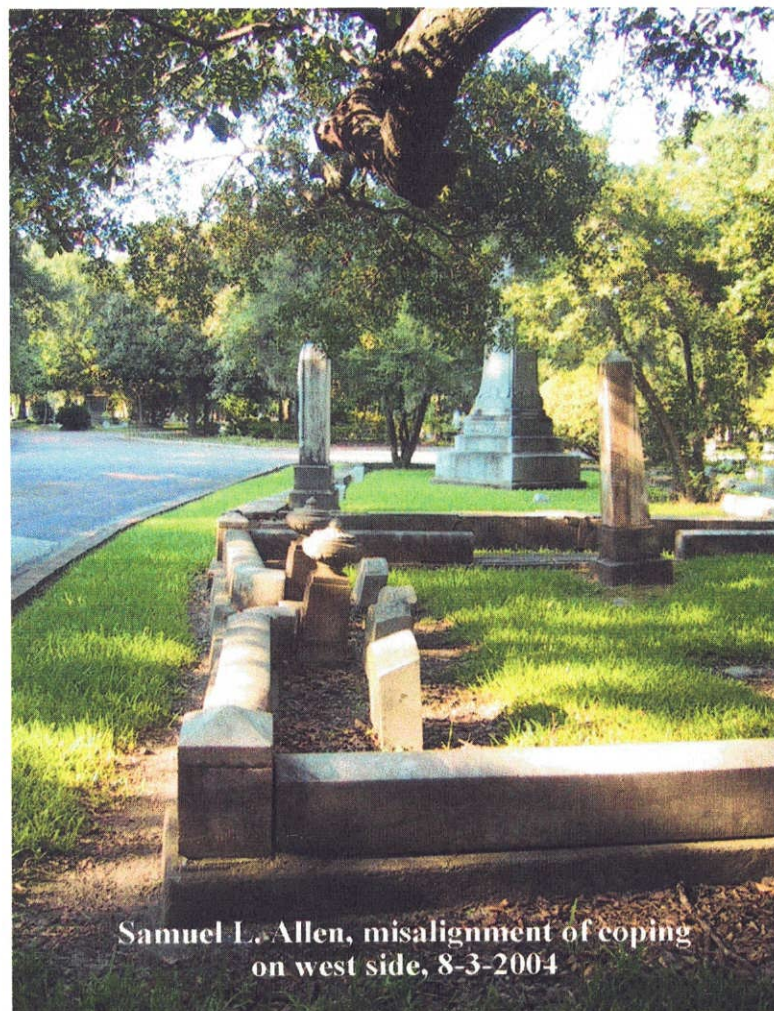
Samuel L. Allen, Section E, Lot 018, fallen coping on north side, 8-3-2004
