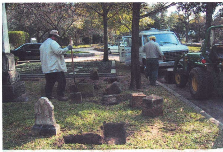
DURING: Excavation proved the lot was marked only by the posts, and there was no coping.
