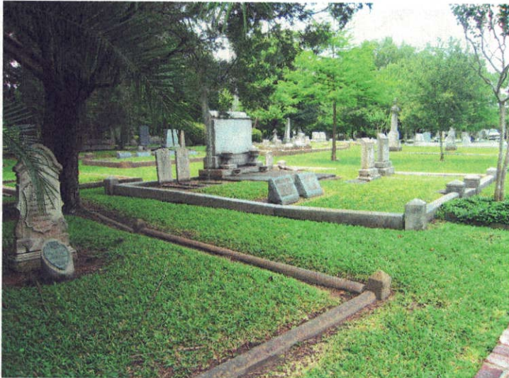
BEFORE: Partially buried cradles are visible in the left rear corner of the lot. The coping is not level and the posts are not plumb.
