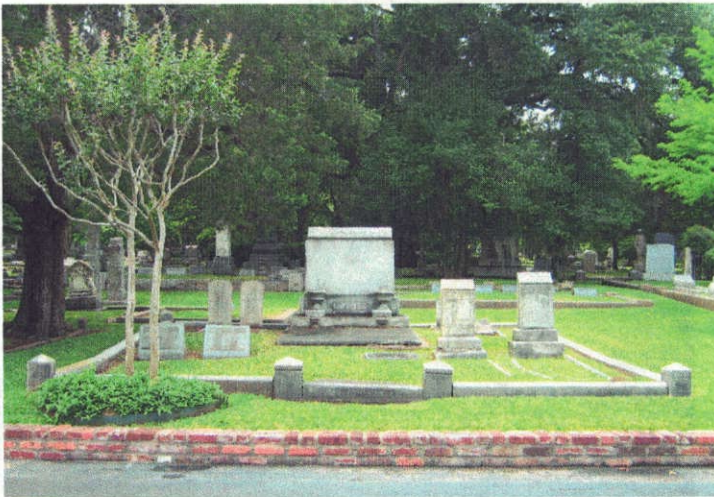
BEFORE: The coping and entrance are tilted and partially buried. Six marble cradles are partially buried, and some markers have been improperly leveled.
