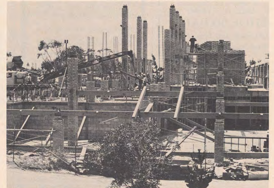
Masons continue their work on the $1 million 21,000 square foot clubhouse addition to the private Lomas Santa Fe Country Club. Architects Lee and Klages A.I.A. of Newport Beach have followed the Mexican Colonial theme of the community in their clubhouse design.
