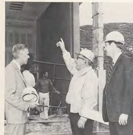
INSPECTION TOUR — Construction superintendent Chuck Allen points out details of Central Federal's new North County office to association President Fred C. Stalder, left, and office manager John D. Pyle. The office, located in Plaza Camino Real shopping center, will open in December.
