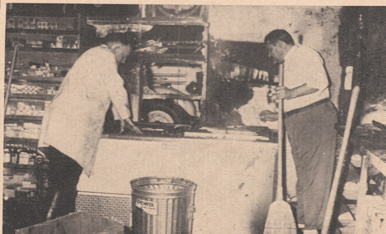
WHERE IT STARTED— Faulty wiring in this freezer unit is credited with starting the fire. Looking over the damage are Fire Chief Jim Fox, left, and Bill Aperance, the owner.
