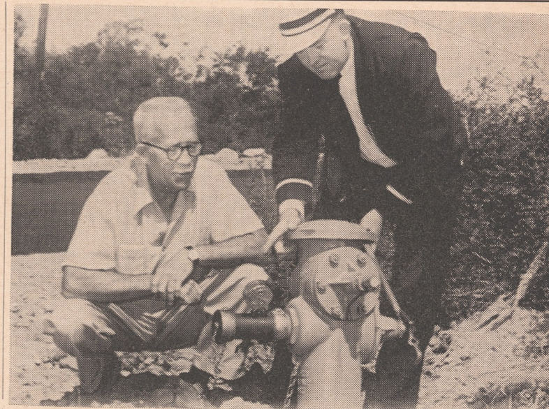
TESTS OK— W. B. Shipway, left is assured by Fire Chief Jim Fox that this regulation type fire hydrant is in good working order. It was installed in accordance with recommendations to all Ranch property owners by both the Santa Fe Irrigation district and the fire district.
