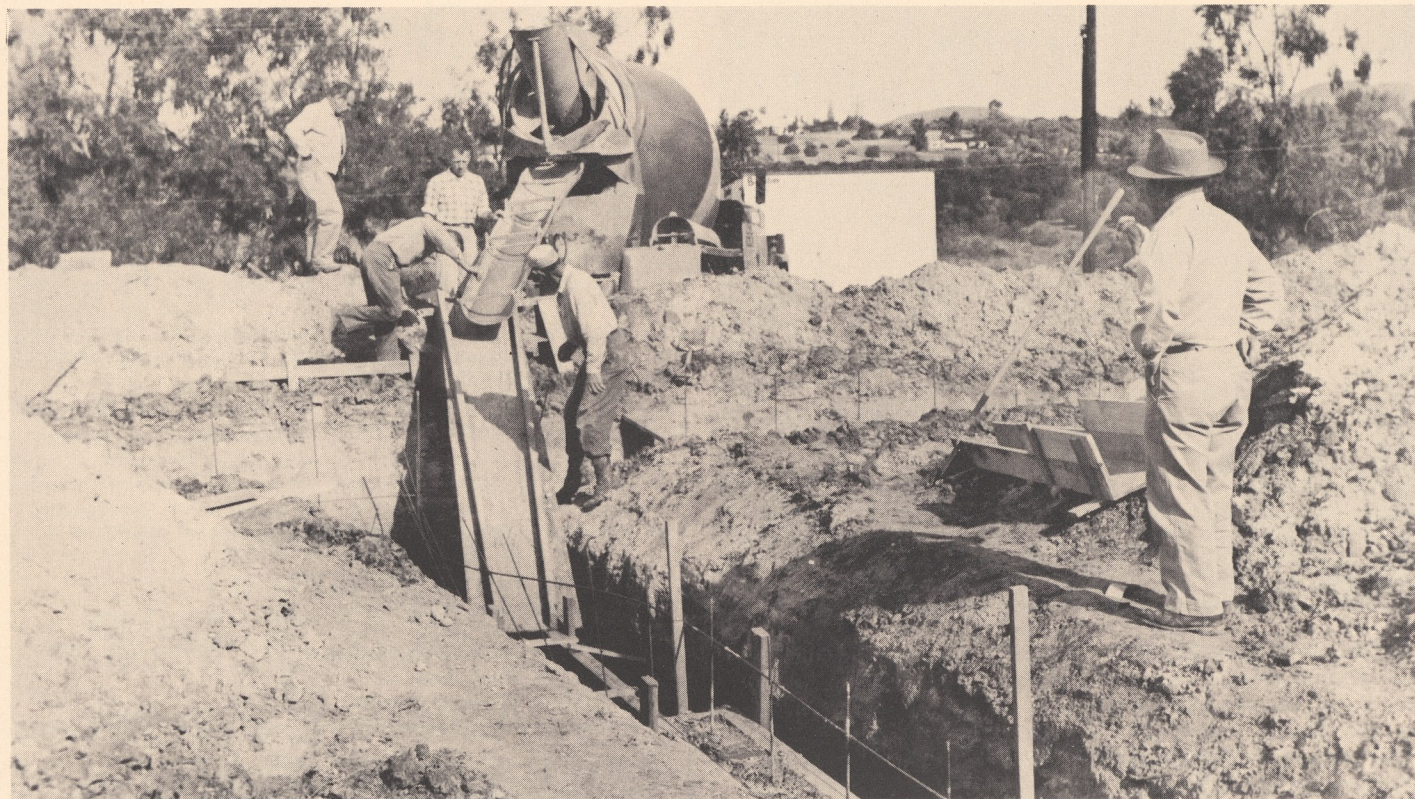
DITCHES AND MACHINERY comprise the scenery on the grounds of the Ranch School these days, preparation for
