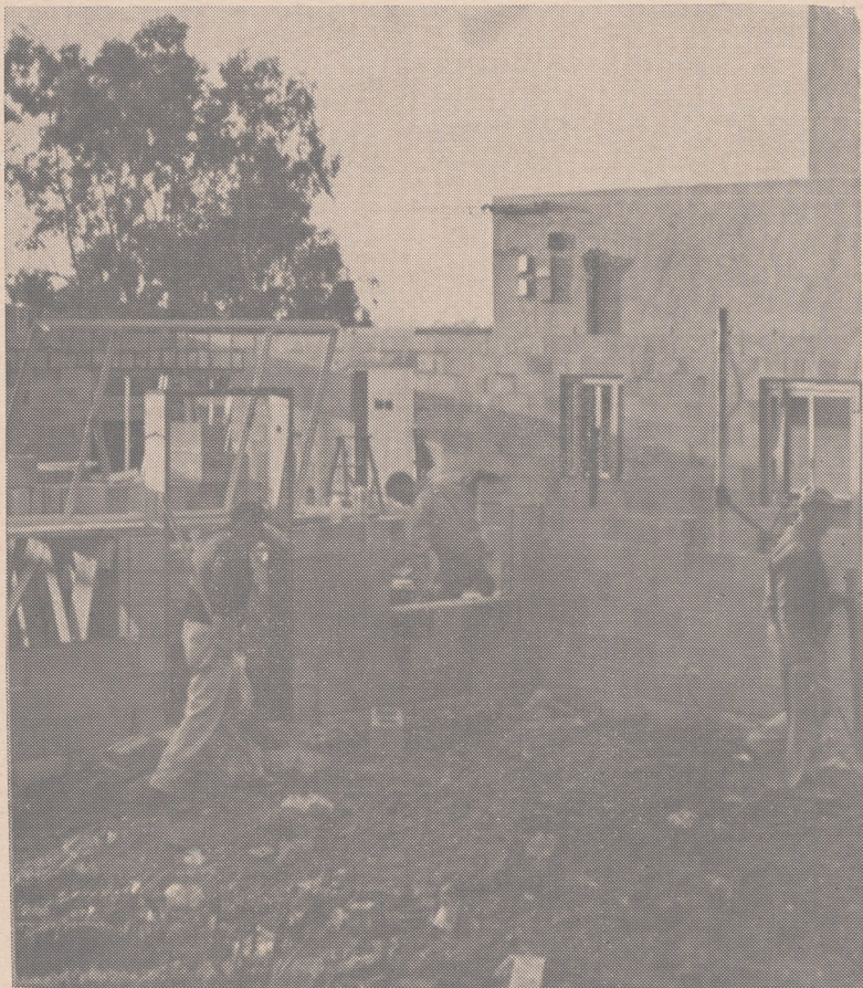
FIRE DEPARTMENT —Construction on the combination Fire Protection District's office and chief's residence is well under way. The building is expected to be completed by at least May 1. The fire department garage is just north of the unfinished structure.
