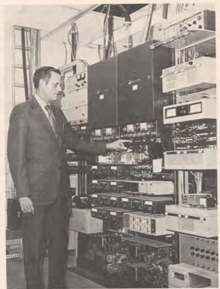
Robert Hively, Director of Communications for San Diego County, is surrounded by microwave transmitters and receivers which allow emergency networks to keep a 24-hour, county-wide vigil over the safety of all county residents. County employees designed and installed emergency mutual aid fire and law enforcement networks as well as emergency medical communications.
