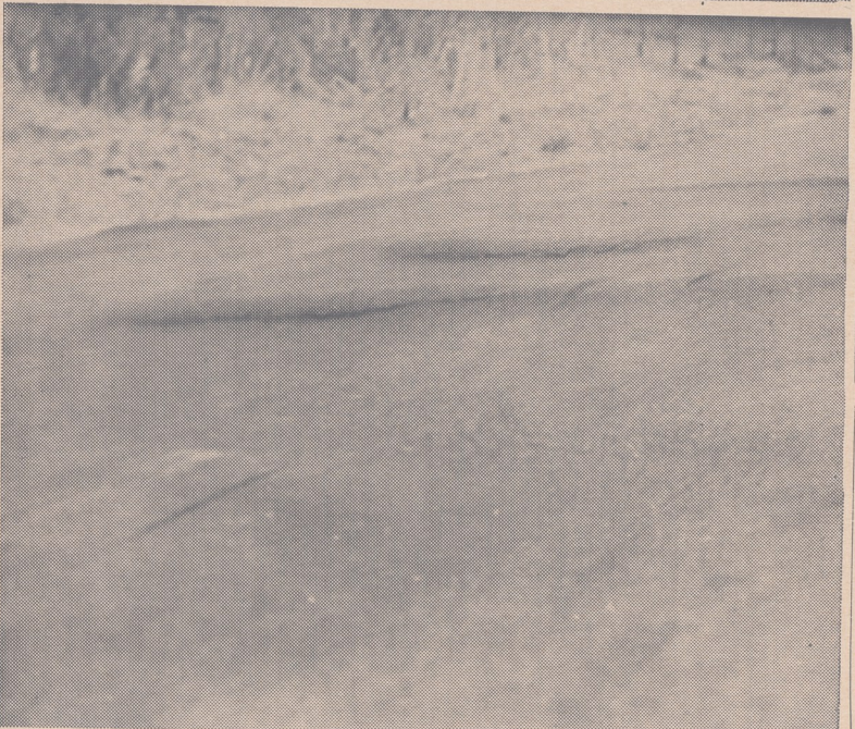
SURF-LIKE SURFACE — These surf-like scenes are located nearly seven miles from the seashore! In fact, it isn't surf at all, but one of the many Rancho Santa Fe roads that are beginning to assume a "rough water" aspect. Deterioration of these roads even more apparent when driving over them than when looking at them through the view finder of a camera, according to the residents of Rancho Santa Fe.
