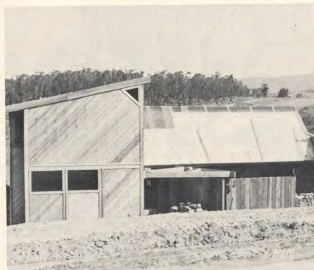
The Tom Hawks home, still under construction. Solar panel faces south and is hidden from general view. Photo by Richard Donnelly.
