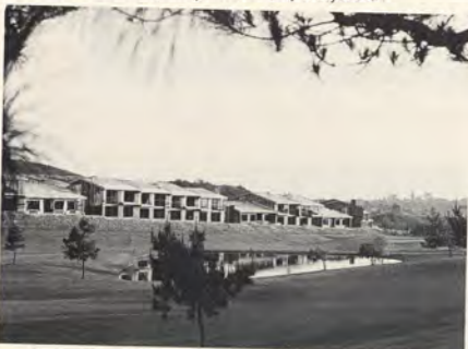
Overlooking the fairways of the Lomas Santa Fe Country Club championship golf course are these two and three bedroom condominium residences under construction at Santa Helena Park. First move-ins are expected about mid-June.
