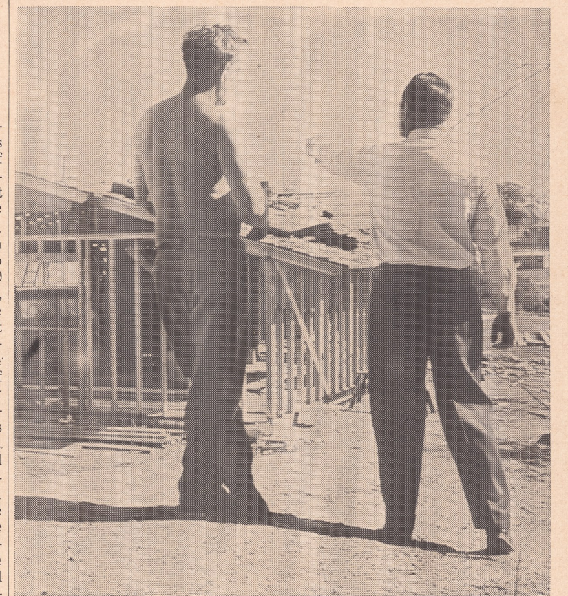
RECONSTRUCTION was well under way this month at the Loma Verde home of Mr. and Mrs. Horace Phillips. Half destroyed by a fire of undetermined origin last November, the Phillips residence now promises to rise like the proverbial phoenix from its own ashes. Mr. Phillips, right, and a builder survey the early stages of this feat from a knoll above the house.
