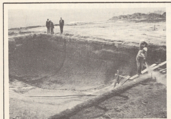
Early last month DEL RANCHO POOLS of Del Mar gunited the huge swimming pool at La Costa Country Club and Spa in La Costa Downs, Encinitas. The country club expects to be in operation by the 1st of May.
