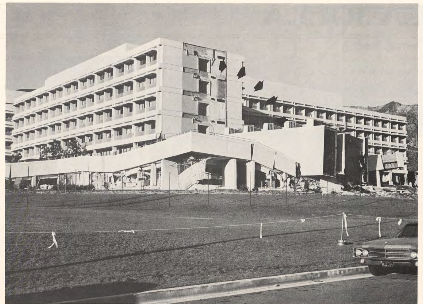
Olive View Hospital, completed only a year before the San Fernando earthquake struck in 1971, was damaged beyond repair. The arrows indicate the movement of what was the stairwell which completely detached from the building and toppled onto the wing below.
