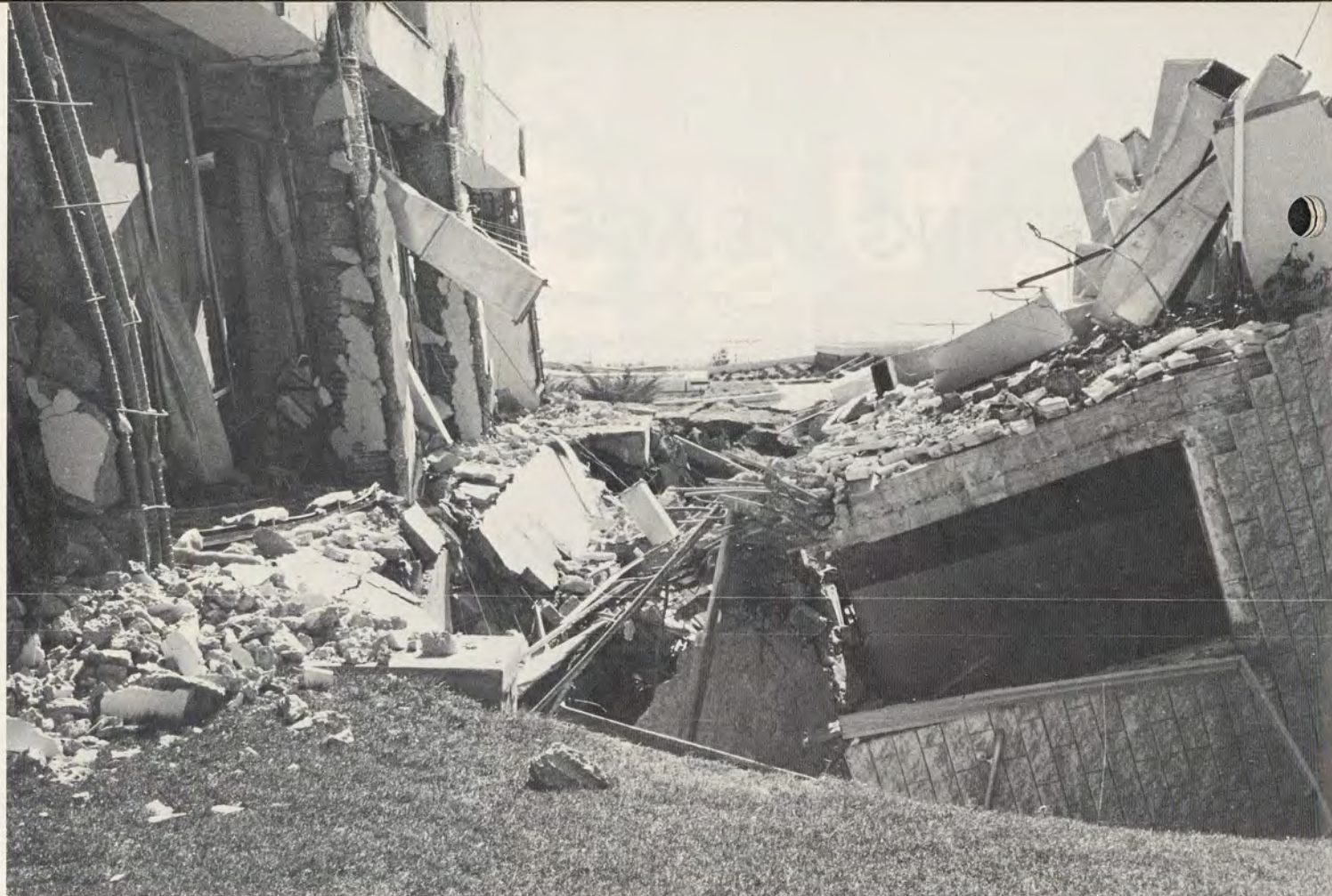
A close-up of the giant section of the Olive View Hospital which detached from one end of the building, toppling onto a one-story section of the building below.
