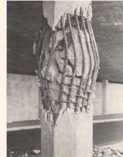
Earthquake damage after the 1971 San Fernando quake to an overpass pillar. This freeway section was built according to the most recent highway seismic safety code.
