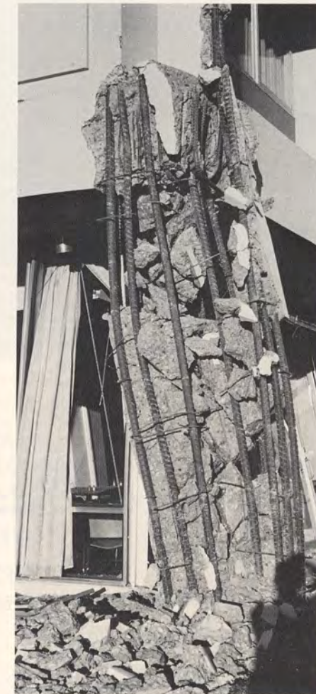
A pillar of the Olive View Hospital. The hospital was built according to seismic safety standards set after the 1933 Long Beach earthquake, yet the building was a total loss.
