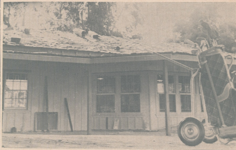
GOLF SHOP RENOVATION added space to the pro shop this month, plus a porch and a new shake roof. Pro shop addition will provide more room for golf carts and equipment.
