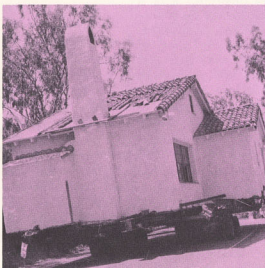
The dining-living room section on top of the grade at Paseo Delicias. Everything going very smoothly at this point.
