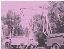
Never let it be said that SD Gas and Electric or Pacific Telephone and Telegram would block progress. Expert crews cleared the wires and cables ahead of the procession and never once interrupted service!
