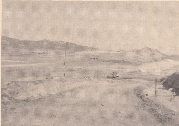
LOOKING NORTH on projected Freeway. Construction continues on 24 hour basis to speed completion.
