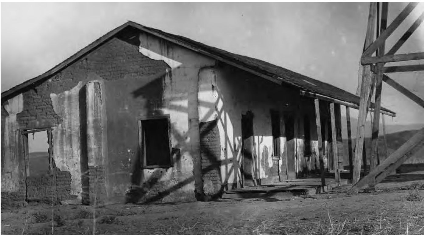
Figure 2.3 Remnant of the Osuna Period of Significance - Rear elevation with water tower and well
