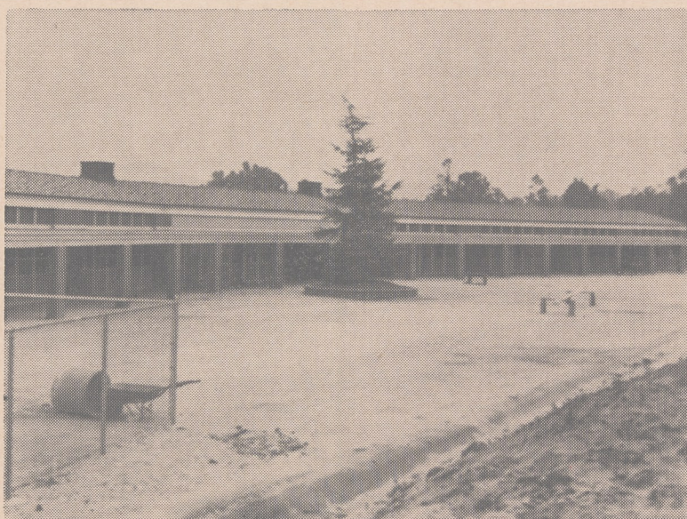
CONSTRUCTION COMPLETED —Youngsters have been in their new classrooms since November 7. The outdoor corridor of the seven-room school follows a trend common to newer schools in warmer climates. Transfer of the 20-foot deodar pine from the old school building was the initial step in the landscaping program. The fenced-in area at the left is the outdoor play area for kindergarten students.
