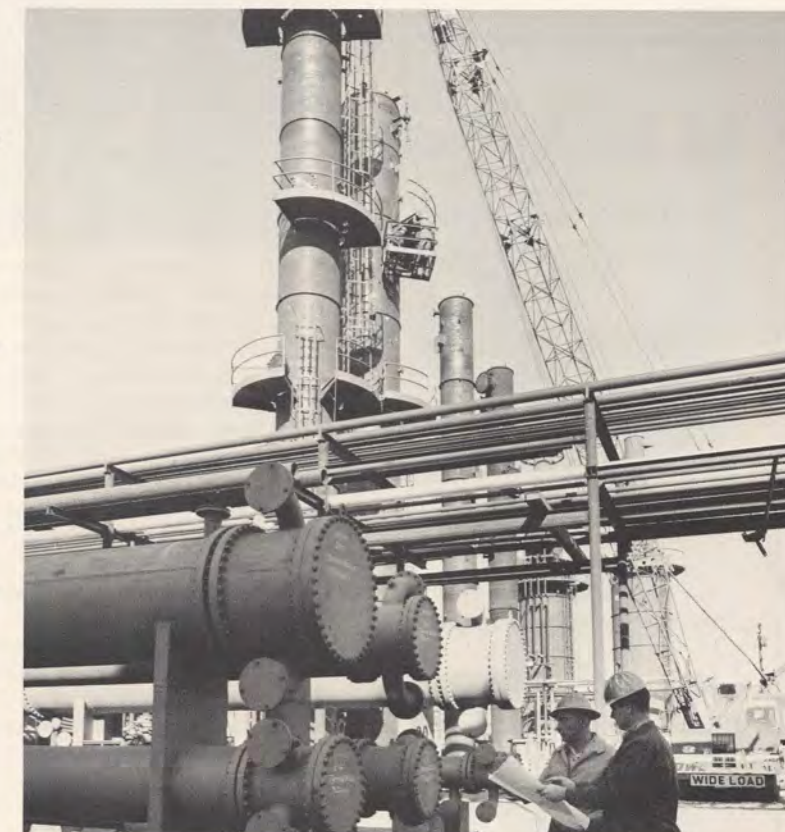
Edgington is currently constructing a new refinery at its Long Beach plant. Scheduled to be "on-stream" by summer 1972, the additional facility will double the firm's throughput capacity.
