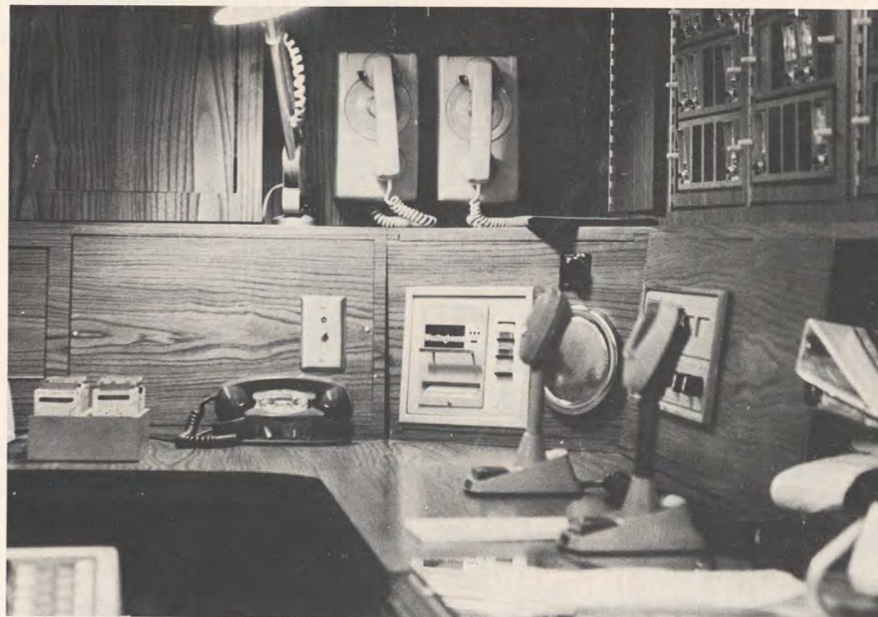
View of the Westinghouse Security System installation at the Rancho Santa Fe Fire Department.
