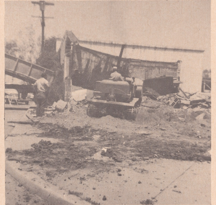
And the Walls Came Tumbling Down as bulldozers razed the old building at the corner of La Flecha and Via de Santa Fe. A new Medical Building will be erected on the site by R. E. Badger.
