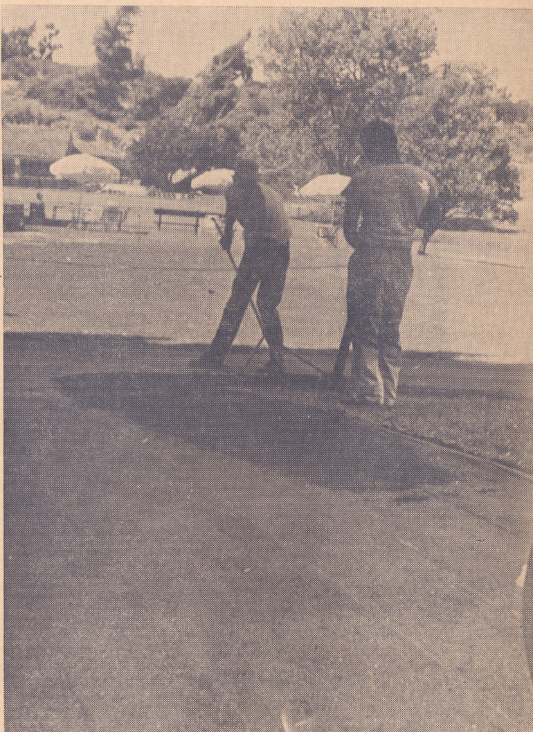
SPREADING ASPHALT on the walkways at Rancho Santa Fe Golf course are employes of Smith Construction company. The asphalt will be covered with fine sand to make the walkway around the course near the pro shop and clubhouse less damaging to the cleats of golfers' shoes.
