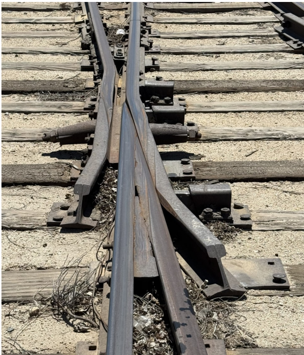
Spring Frog on the main line at the Campo Depot
