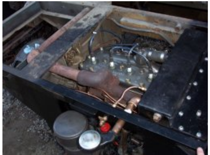
The Enginator with the generator on the left.
