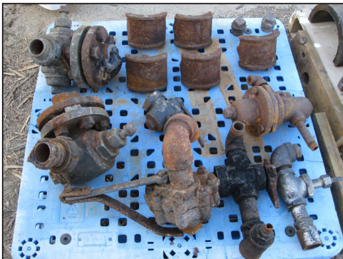
Boiler check valves and other parts.
