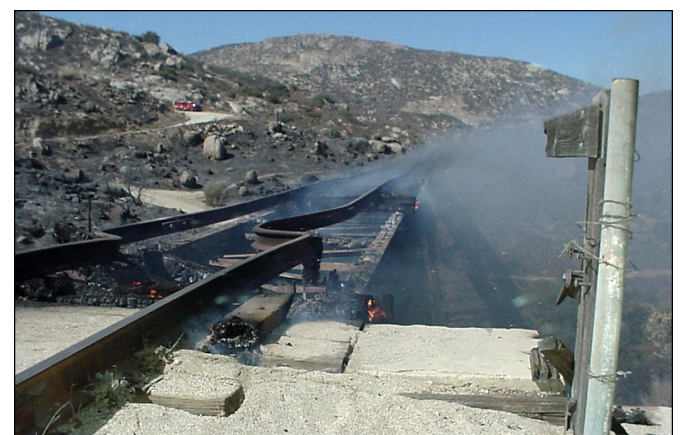
The west pier of the Lower Campo Creek Bridge all but consumed. Photo courtesy International Border Rail Institute
