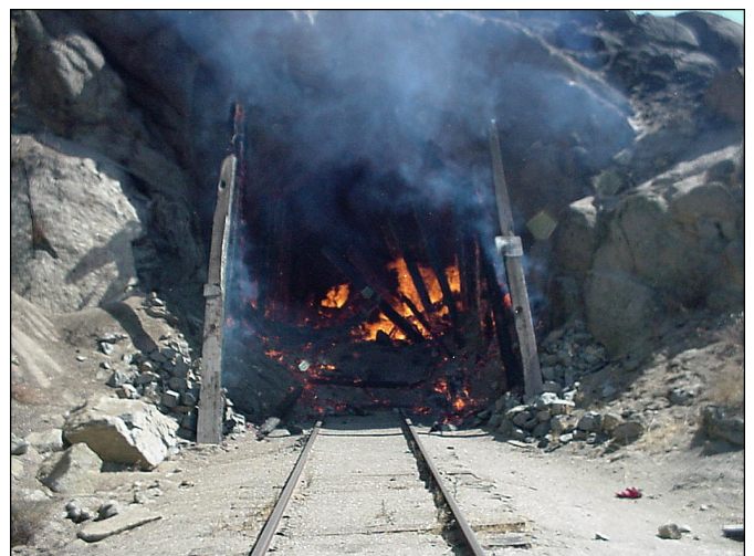
The east portal of Tunnel 4 still burning.
