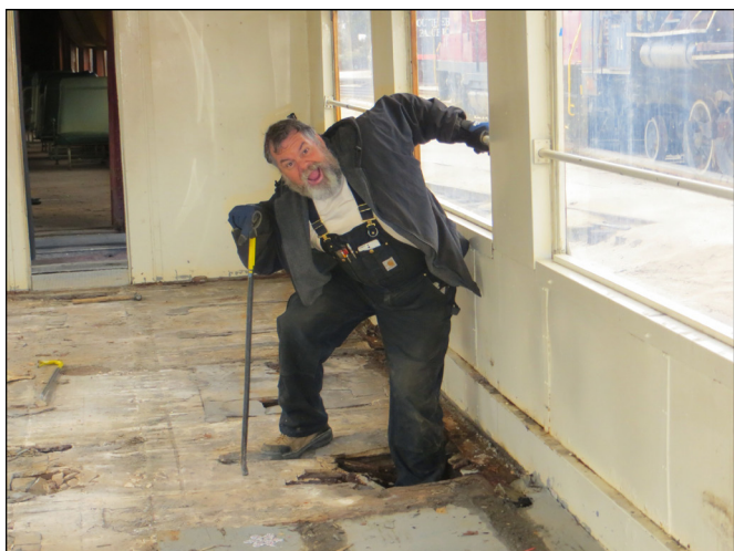
Rusty Hoar discovers the floor of the 350 is in worse condition than originally thought. Ron Hyatt Photo
