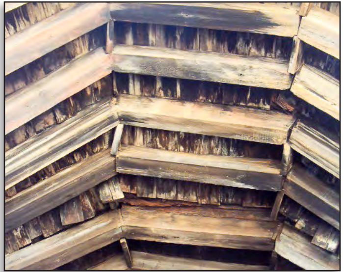
West portal roof timbers showing deterioration.
