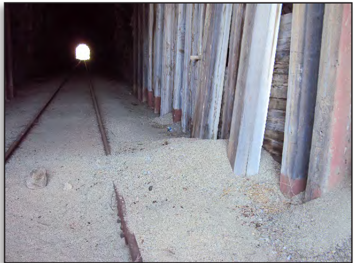
Erosion at the west end of Tunnel 4.
