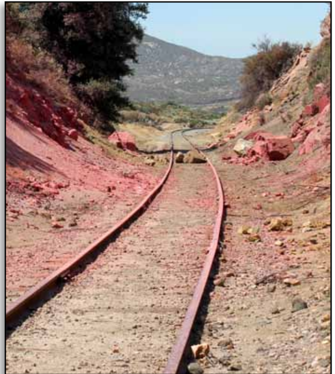
Fire Retardant covers the tracks at the Milepost 63 Cut. Notice the two large rocks in the gauge.
