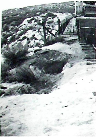
This close up at the railroad east end of the bridge shows the need for repairs as the embankment had washed almost under the tracks
