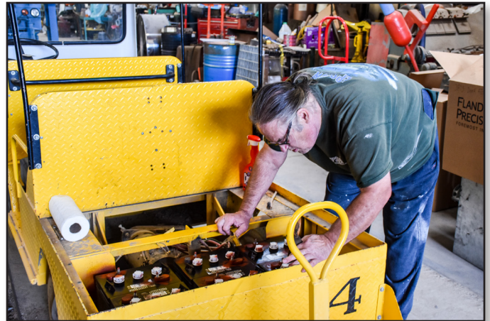
Charles Smith maintains the batteries on one of our electric carts.
