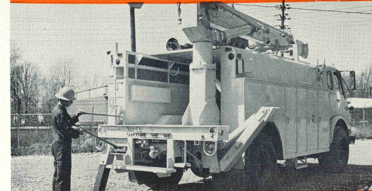
Operation of the line truck's equipment is achieved with 36-inch fiberglass handles. Note that jack location has been moved substantially forward.
