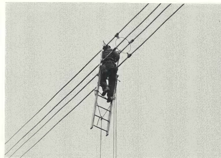
Bundle spacers are attached at 250-foot intervals. Spacer consists of loop of stainless steel wire with conductor clamps positioned at 90° intervals to maintain 18-inch square configuration.
