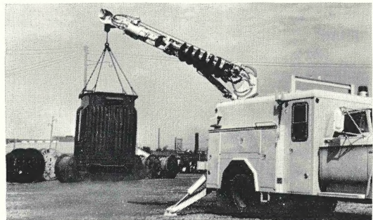
SOLUTION: Override the overload device, elevate boom, lower with winch line.
