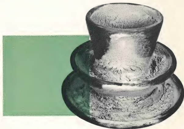
69-kv Multipart insulator after about three years of exposure near a cement plant. A prior application of silicone wax, as discussed in the paper on surface leakage, would have made removal of these deposits much easier.
