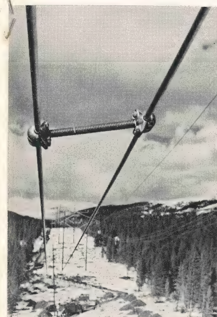
9. A helical spring spacer on the two-conductor bundle. All spacers, like the control rings and clamps, were tested before installation to make sure their critical corona voltages were equal to or better than the conductor.
