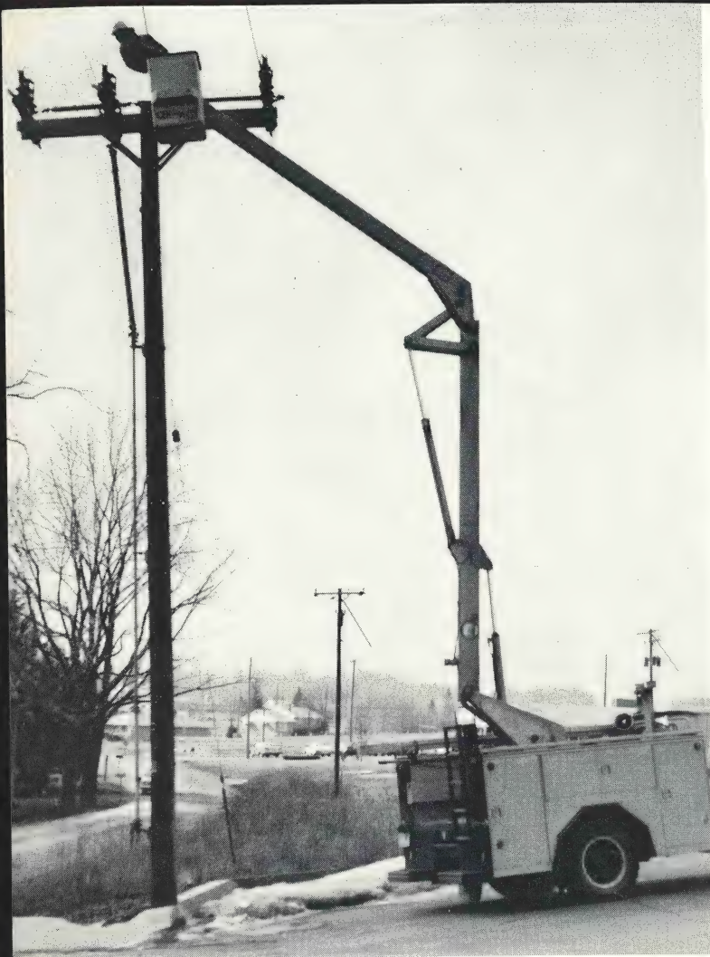
Check-out of 12470-volt shopping center feeder line uncovers burned connectors before they've caused television interference or power outage.
