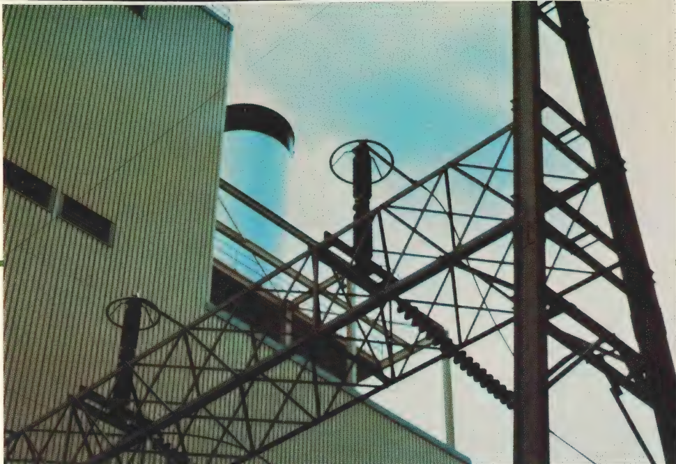
Among SPS firsts is the installation of O-B's new DynaVar surge arresters with metal-oxide varistors for station protection.
