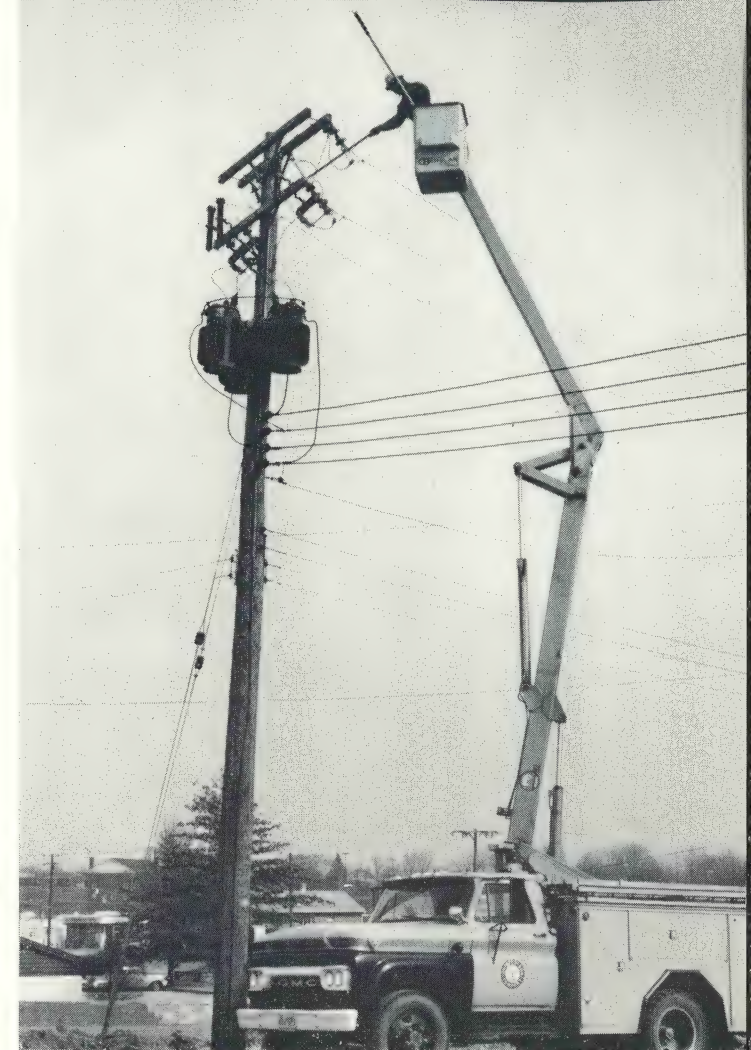
Serviceman in aerial bucket checks for loose connections in pole hardware, using a switch stick.
