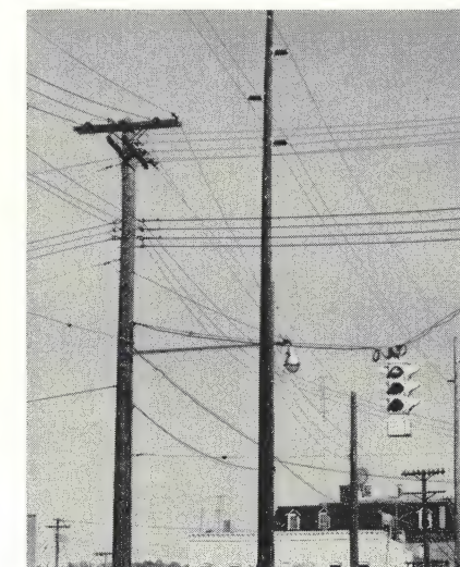
(B) Note the considerable saving of space offered by horizontal posts in this 69-kv circuit; occupying less width in right-of-way than the 4-kv feeder beside it.
