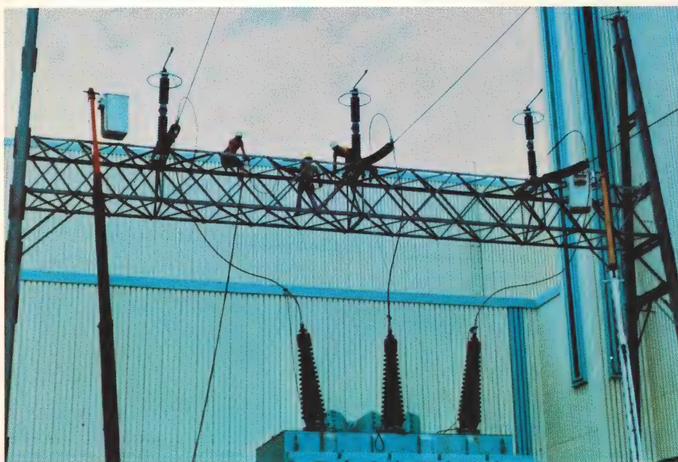
An SPS crew installs three of the nine O-B DynaVar arresters used to protect transformers at Clifford B. Jones Station, Lubbock, Texas.
